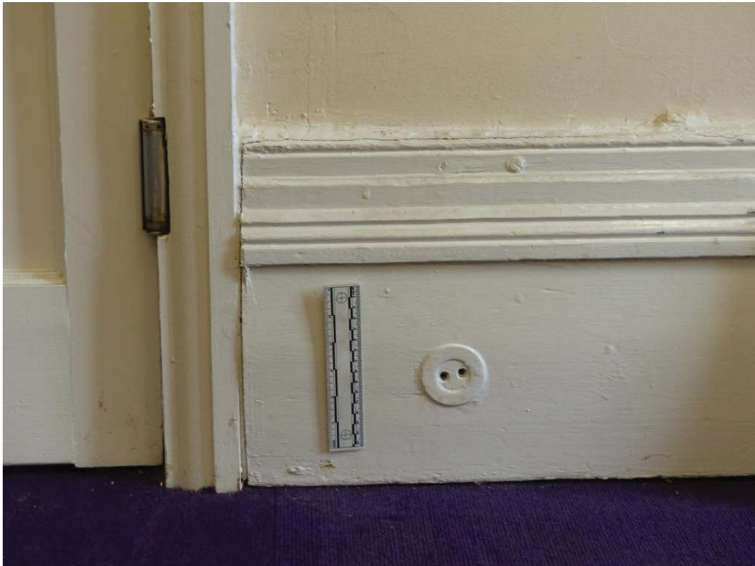
Fig 64 The early electrical socket in the north wall of room G3, looking north
