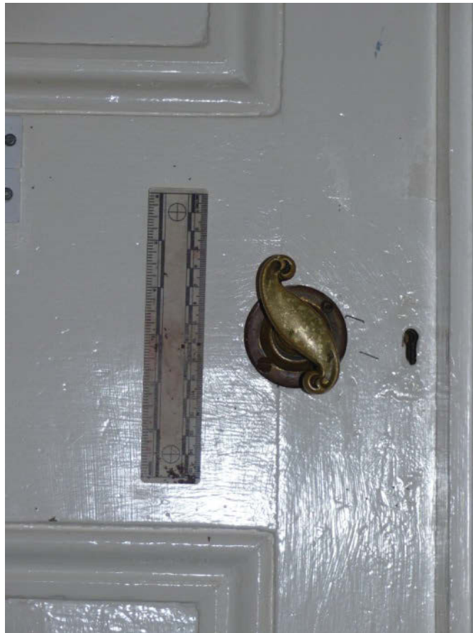
Fig 87 The door handle of the obsolete door to the former northern part of 1F3.
