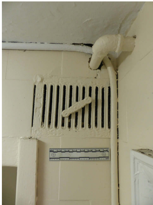
Fig 69 The air vent in room G11, looking south. Note the glazed tiles painted over
