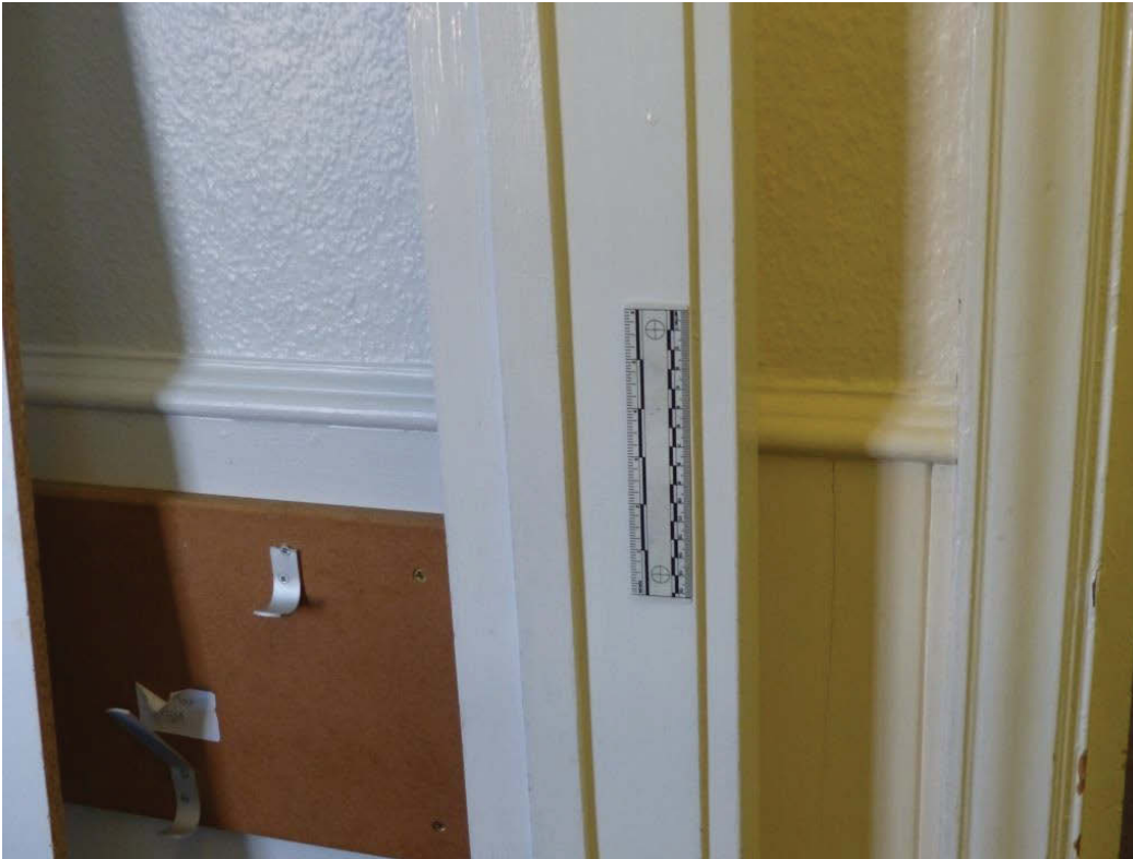
Fig 68 The dado rail running from the corridor G9 into room G10, interrupted by the modern door frame, looking south
