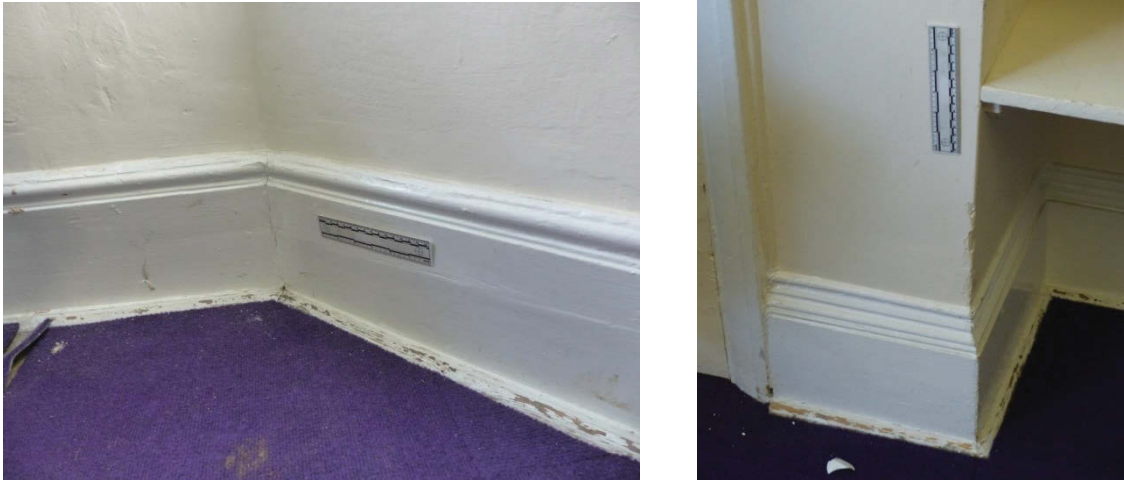
Fig 67 Variations in the skirting board in room G6. The earlier example from the bay window area is on the left, with the later example from the former fireplace on the right.
