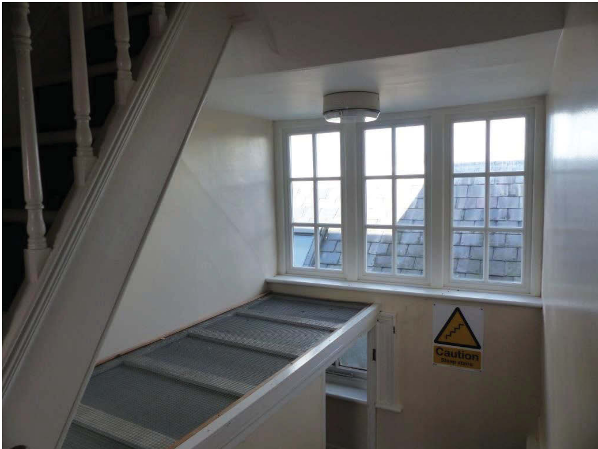
Fig 79 The view of the staircase area at 2nd floor level looking north-west. The original, two pane window is at bottom-centre. Note the diagonal scar on the wall, indicating the line of the former roof pitch. Steps up to the attic water tanks are on the left.
