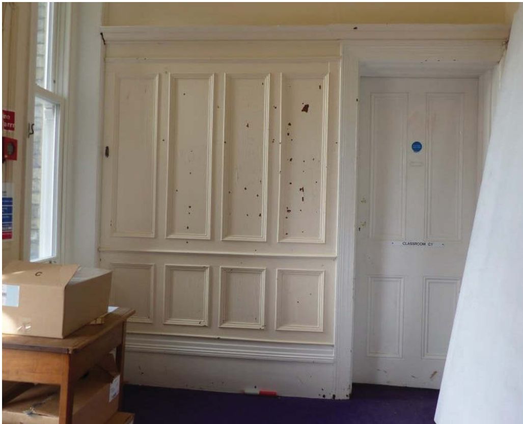
Fig 57 A section of panelling in the south west corner of room G1, looking west
