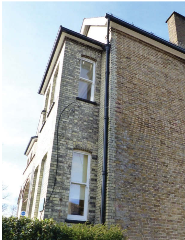
Fig 24 The south-west corner of Claremont, looking north-west, showing the bond between the Gault and stock bricks.
