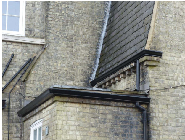
Fig 33 The decorative brick cornice below the eaves of the gambrel roof, north façade, looking south-west
