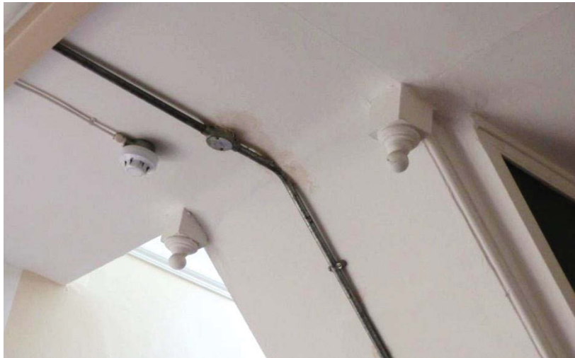
Fig 77 Two spherical pendants in the ceiling at 1 st floor level, looking north-west
