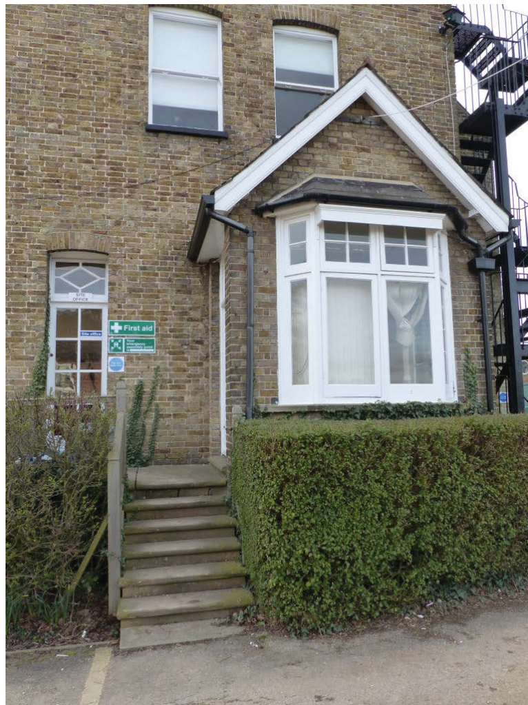
Fig 25 The narrow ventral door and box-bay window in the east façade, looking west
