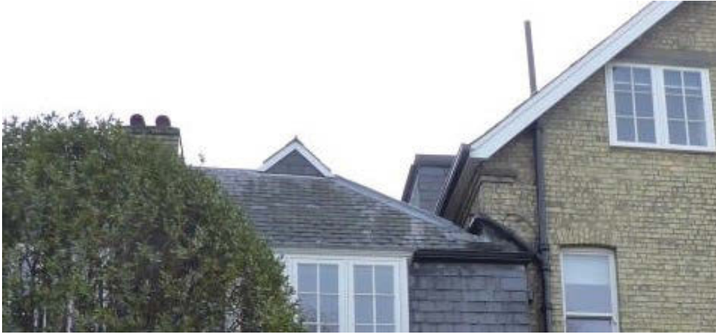
Fig 44 The gablet of the Phase 2 roof, visible above the ridge of the later Phase 3 gambrel roof, looking east
