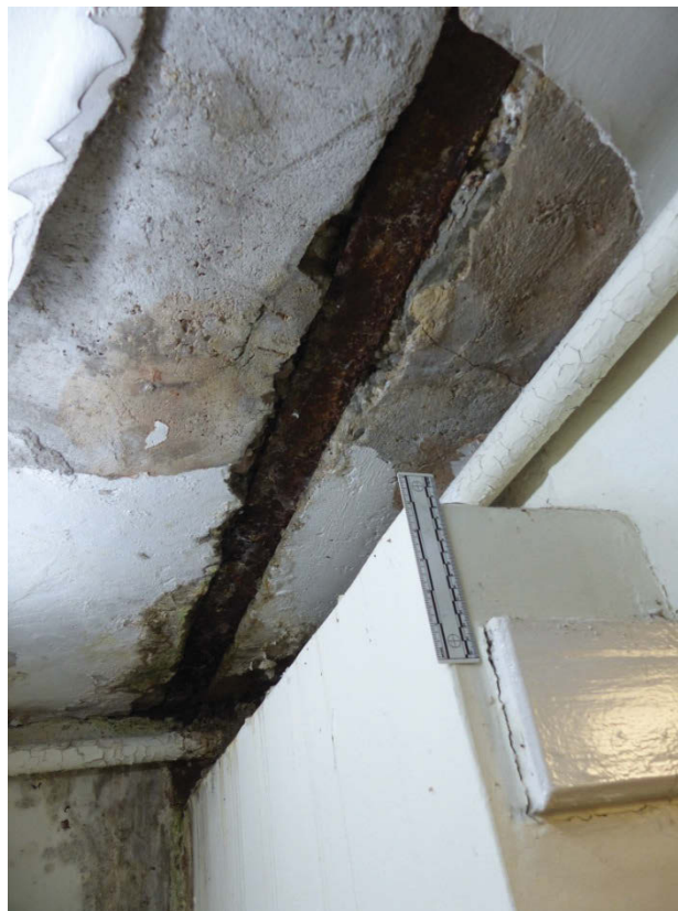
Fig 47 The wrought iron band exposed in the ceiling of B1, looking south
