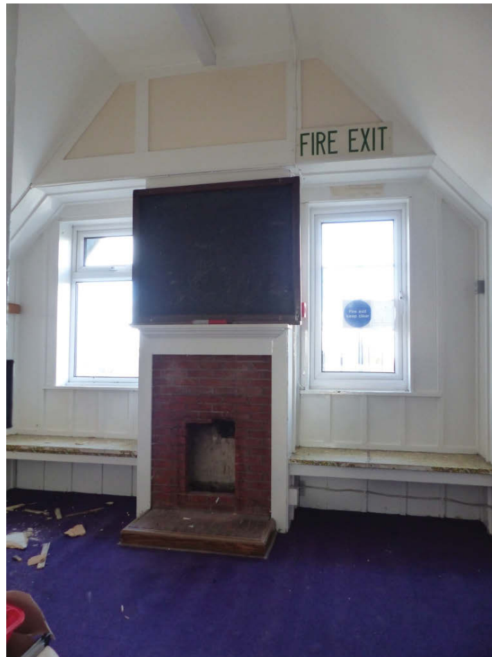
Fig 102 The windows and fireplace at the north end of room 2F4 looking north.
