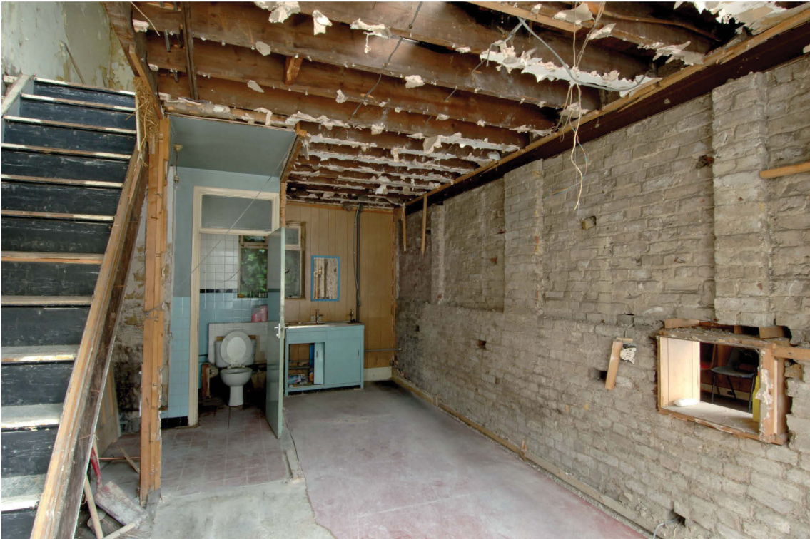
Fig 8 Internal view to east of ground floor of building at east side of site
