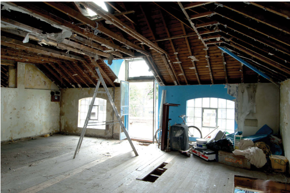
Fig 9 Internal view to west of first floor of building at east side of site
