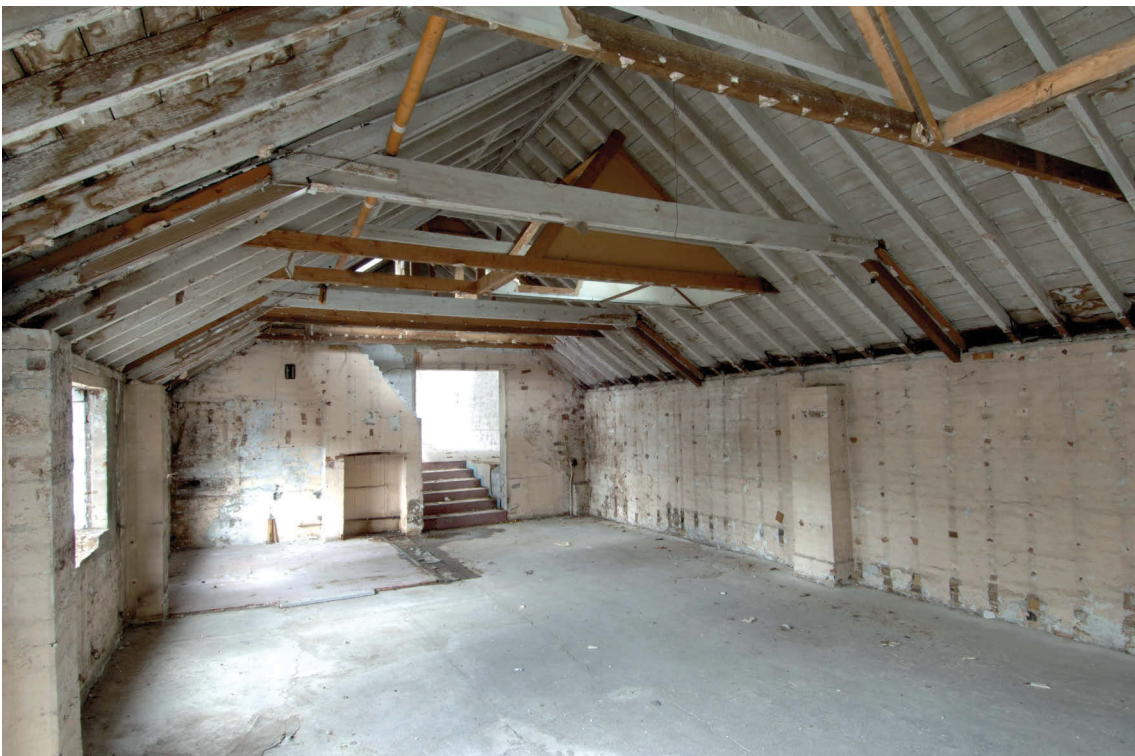
Fig 13 Internal view to south of first floor of building at west side of site
