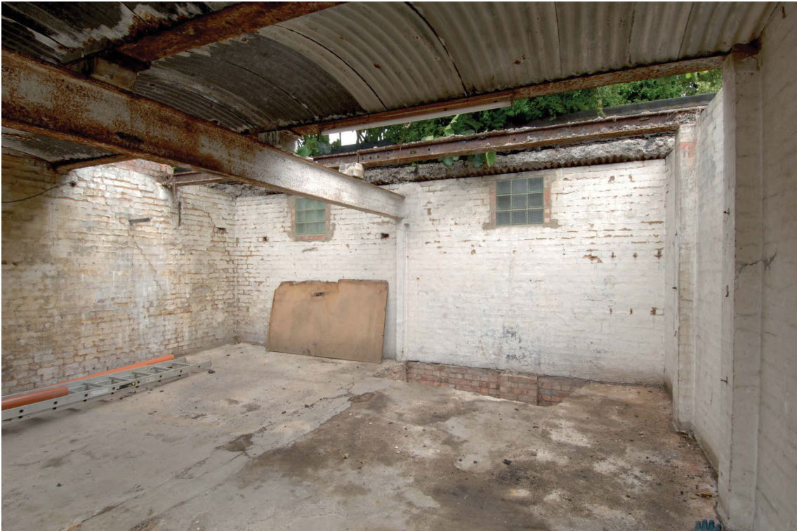
Fig 10 Internal view to southwest of building at southwest corner of site with poured concrete ceiling slab above arched corrugated iron sheets
