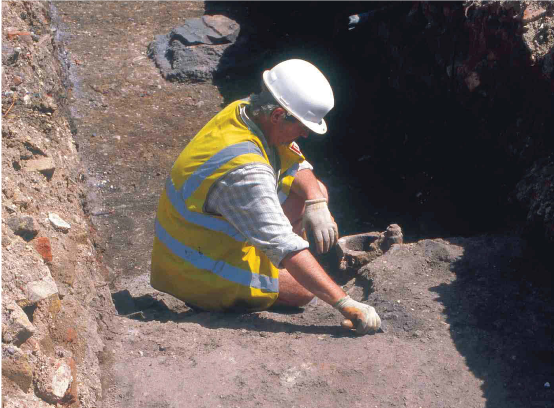
Fig 20 Trench 1B, crushed cinder floor of Paxton's Tunnel (46) with iron column (44) and joist support (37), looking east
