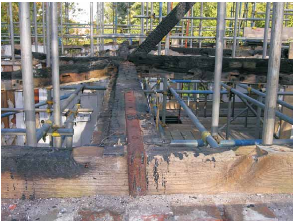
Fig 35 West end of wall plate on the main internal wall, strappes to plate on external wall, looking east
