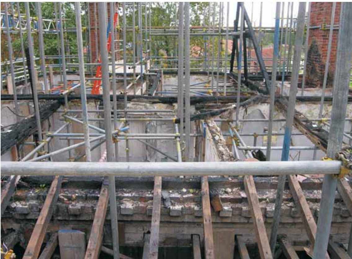
Fig 33 Dentilled brick eaves of the original external north wall of the cottage (foreground), to which a lean-to extension was later added, looking south
