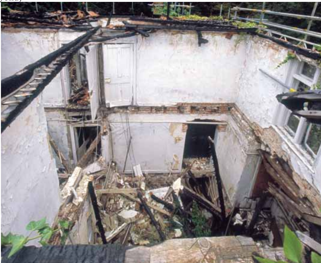
Fig 27 Looking north at eaves level into IF3 and G10, with B1 and B2 visible below
