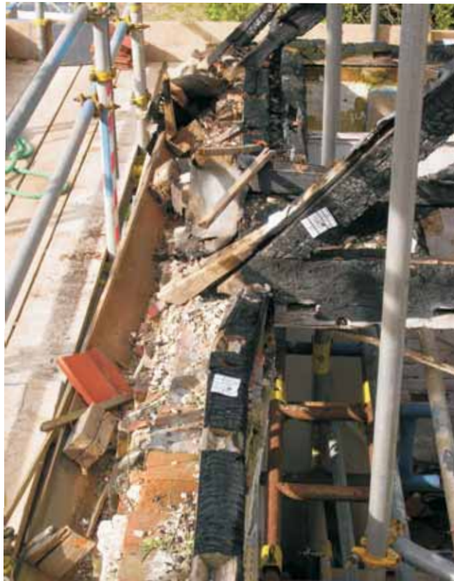
Fig 39 Wall plate on south external wall, broken where it has been pulled north by a tie-beam over IF4, looking west
