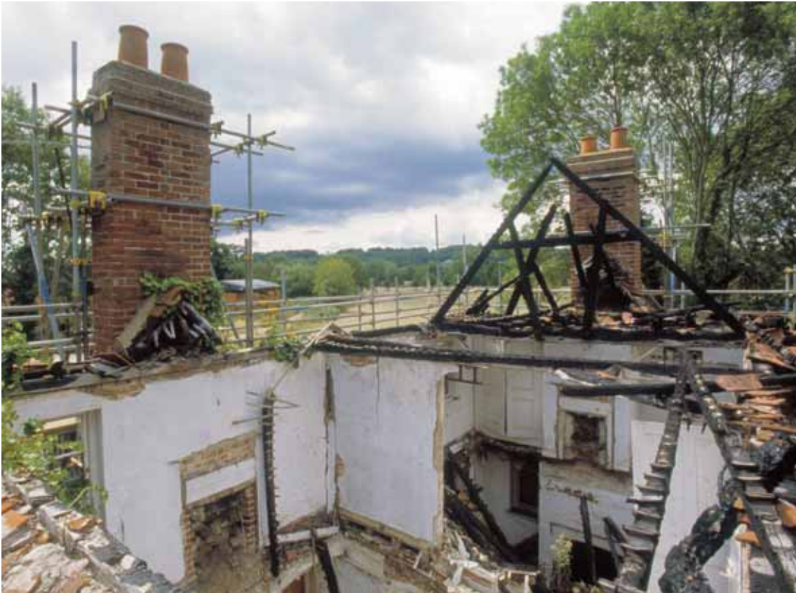
Fig 24 Looking south-west at eaves level into IF3 and IF4. The roof truss was the only major group of roof timbers still in situ
