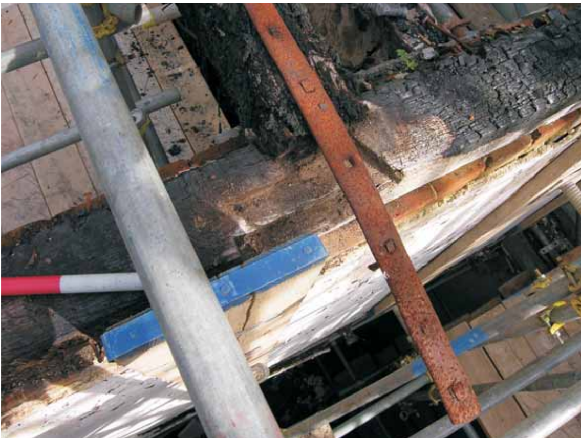
Fig 37 Iron strap across central wall plate, nailed to tie-beams to north and south (the latter burnt away), looking north-east
