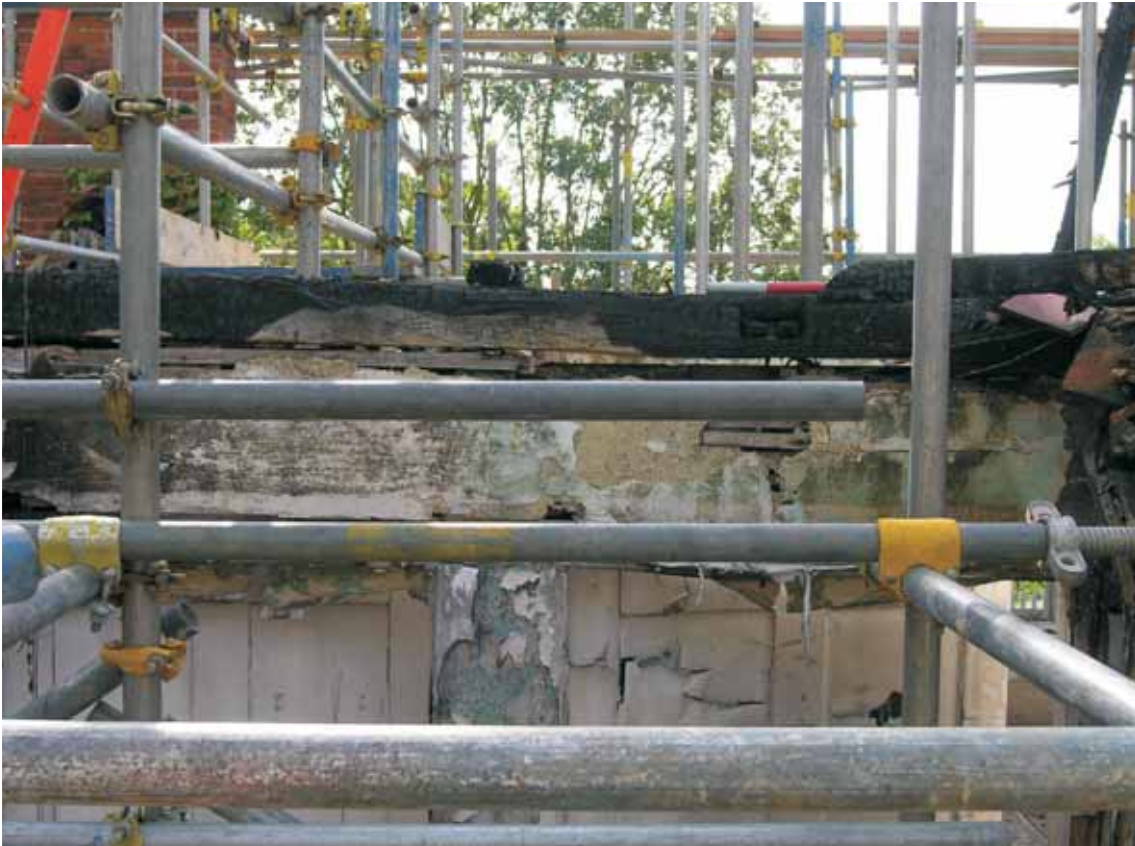
Fig 36 North face of internal wall and wall plate in IF1, looking south
