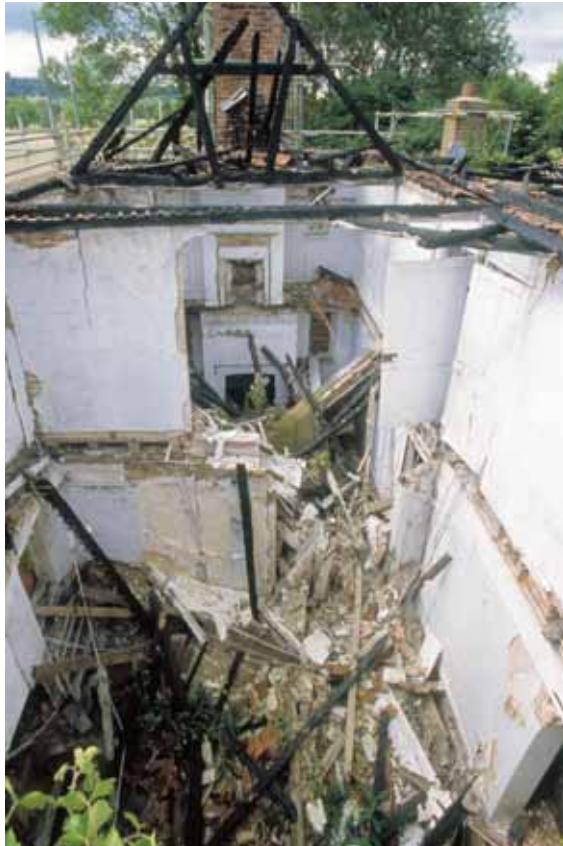
Fig 26 Looking west at eaves level into IF3, G10 and B2 (below), and IF4 and G2 (beyond)
