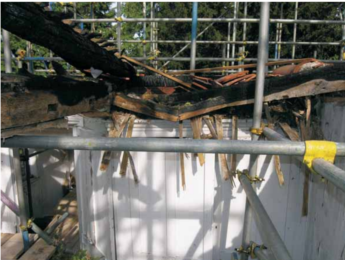
Fig 31 Partially collapsed roof remaining over IF5, looking north
