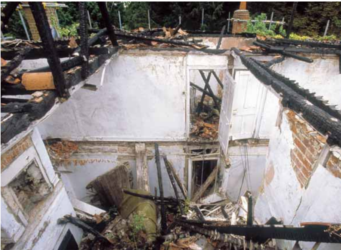
Fig 25 Looking north at eaves level into IF4 and G2. The stud and brick north-south partition wall had partially collapsed
