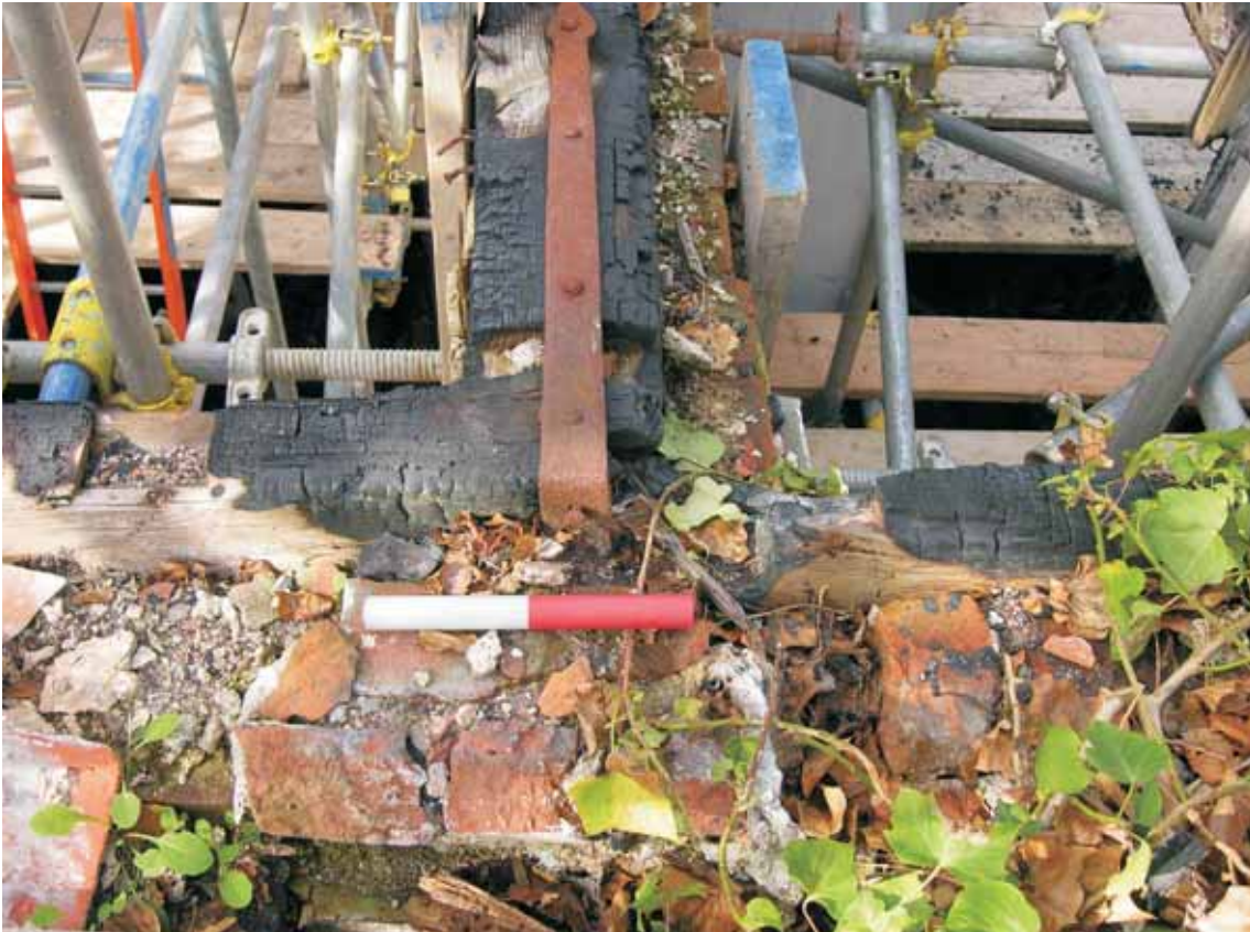
Fig 38 East end of central wall-plate, strapped to the plate on the external wall. The latter wall has moved outwards, breaking the wall plate on it immediately to the north of this joint
