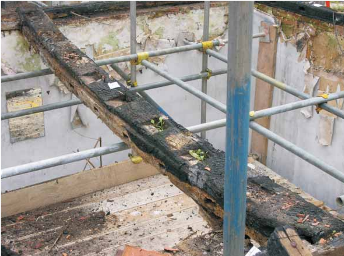
Fig 34 Detail of empty joints for seating rafters in a tie-beam over IF5, looking south-west
