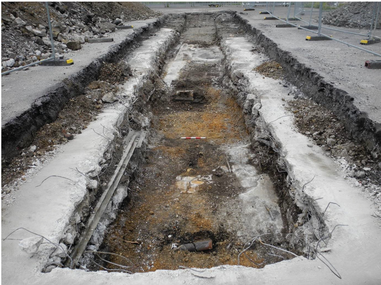
Photo: brick sumps and the railway track to the south (left), Trench 2 looking west
