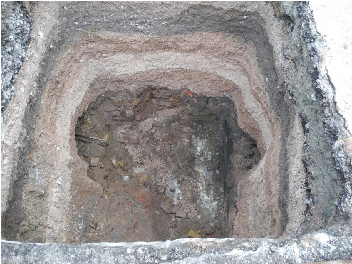
Fig 4 Photo; Trench 2 showing the concrete below the partially removed brick foundation, the remains of the iron girder to left and the modern pink deposits, looking west
