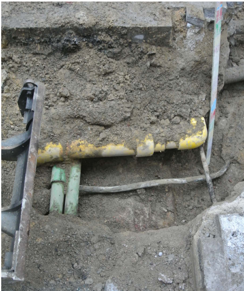
Plate 8 ST3, drain or sewer [11] partially exposed in the base of the trench. Looking east
