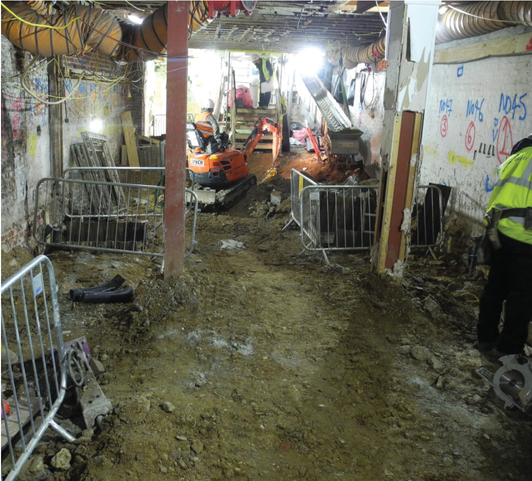
Photo: the current basement showing some of the columns before the ground reduction (looking SW)
