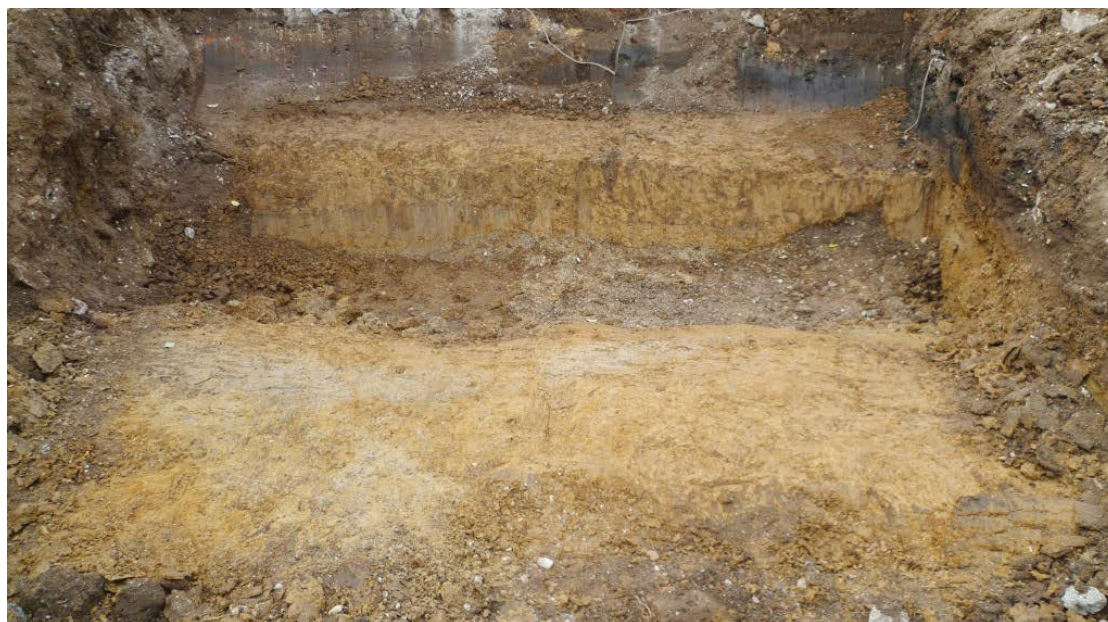
Photo 1 looking west, showing extension of the west area with alluvium truncated by pad foundations
