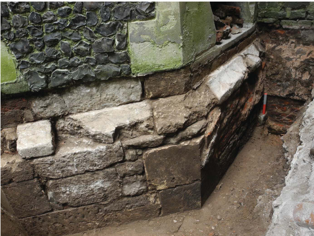
Photo 18 Face of original Tudor tower exposed with later knapped flint face, looking east
