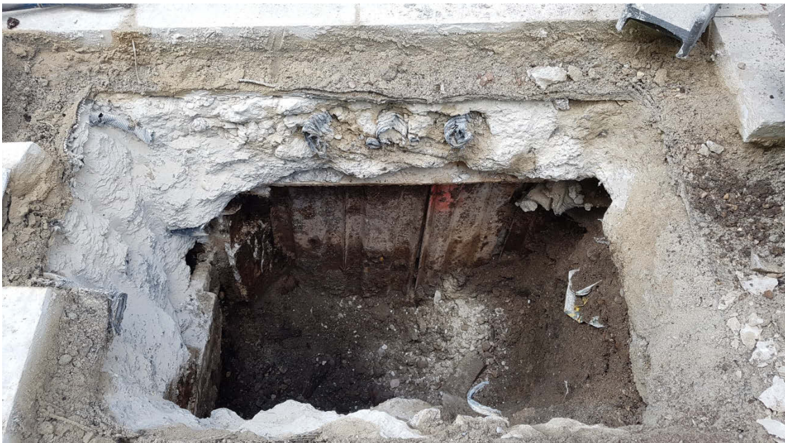
Trench 1B showing reverse of sheet piles at side of GUD99 excavation trench, with bulk backfill [6] in modern sewer construction trench in foreground (looking west)
