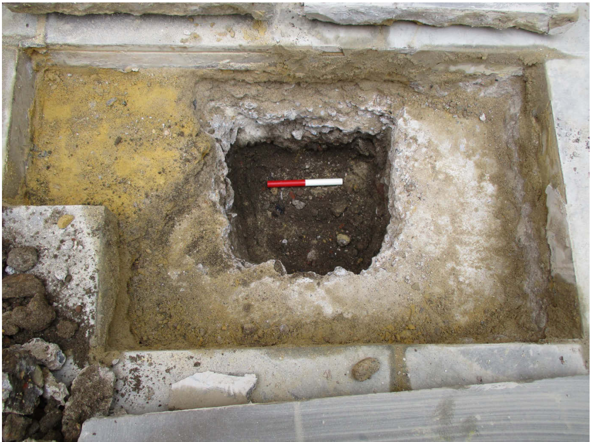
Test hole 2A showing soft deposits [7] exposed beneath concrete slab looking east (0.2m scale)
