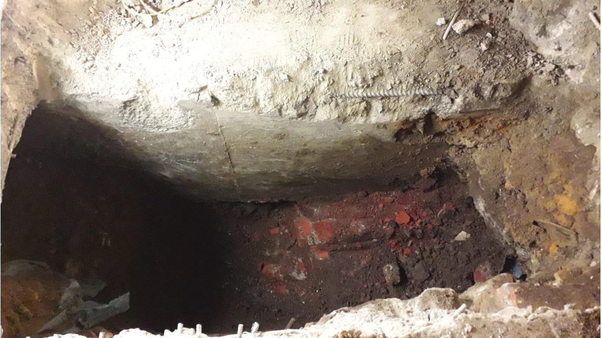
Photo 1 TP1 looking NE showing 18th century brick wall [9] partially under 1990s ground beam
