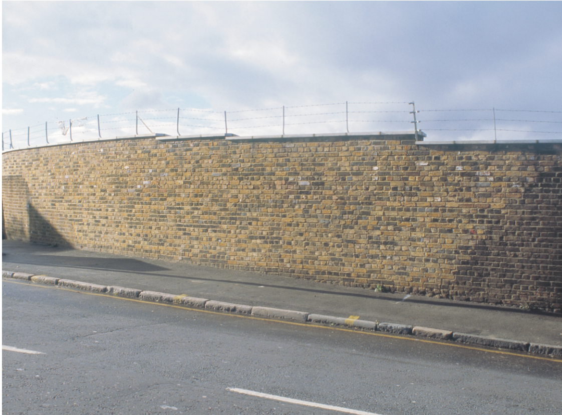
Fig 13 Repaired section of the wall on the site of the former Hydraulic House, looking west
