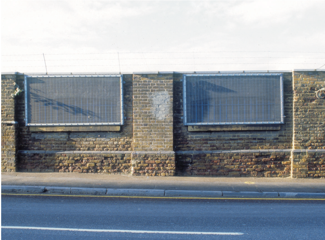
Fig 11 Blocked window openings in the wall of the former Brass Foundry, looking west
