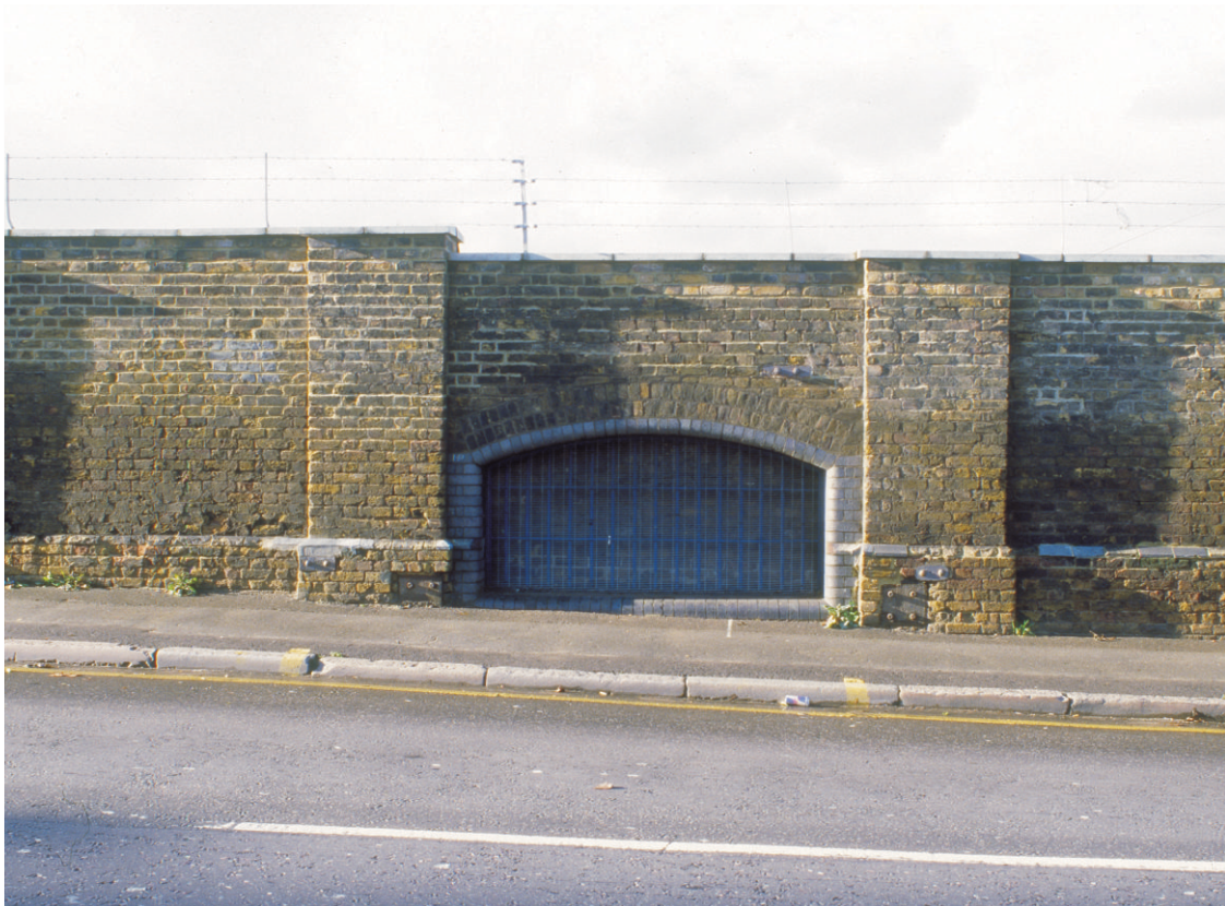
Fig 12 Blocked window opening lighting a room below street level in the former Brass Foundry, looking west
