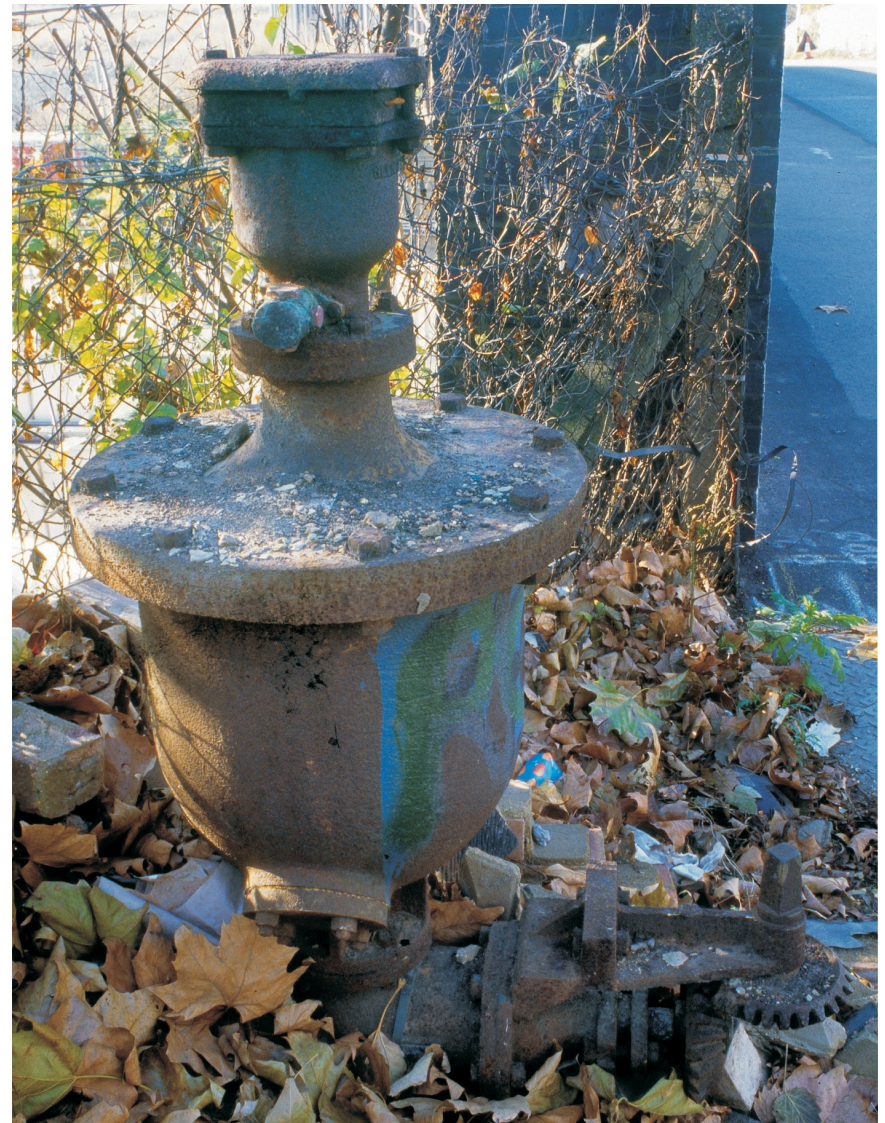
Fig 7 Air valves mounted on horizontal isolating sluice valve, looking west
