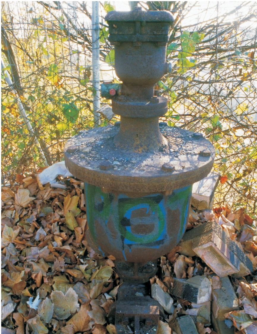
Fig 6 Small and large orifice air valves mounted on horizontal isolating sluice valve, looking south
