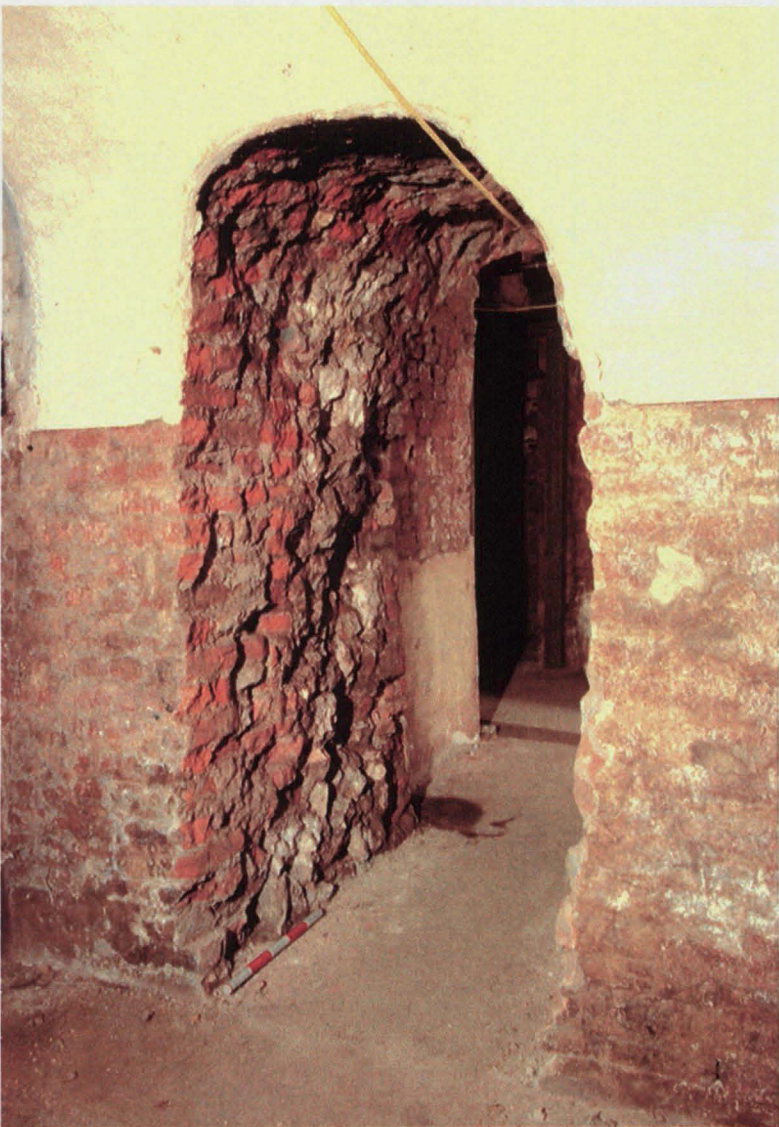
Fig 17 North wall of southern passage below western and eastern cellars, looking northeast
