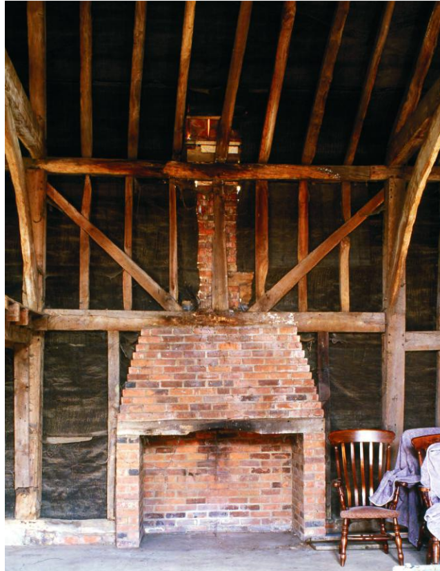
Fig 14 The fireplace inserted into the north wall of Phase 1 of the barn
