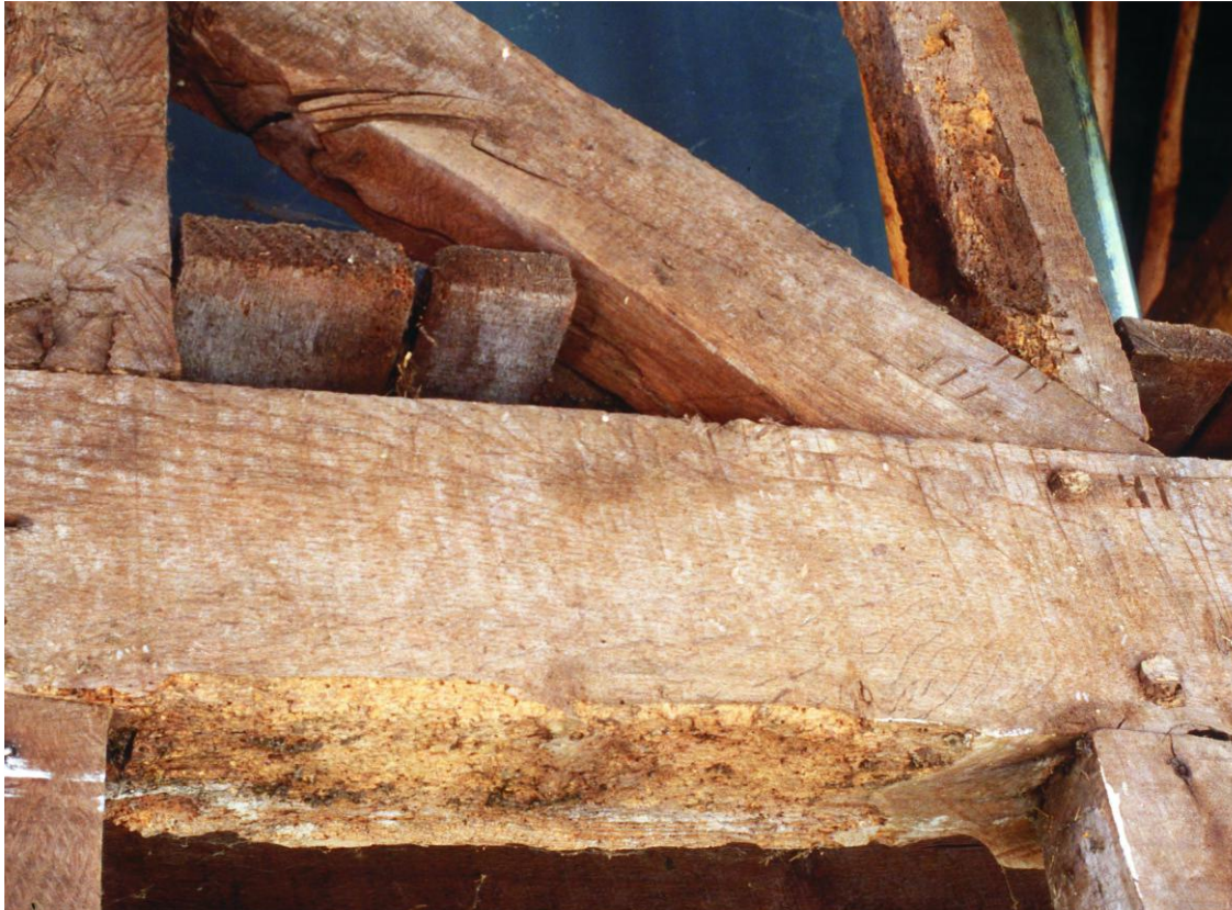
Fig 16 Carpenter's marks on a midrail and studs in the south wall of phase 1 of the barn
