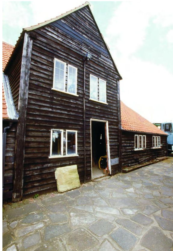
Fig 9 The wagon entrance and catslide roof in the south-facing facade of the barn
