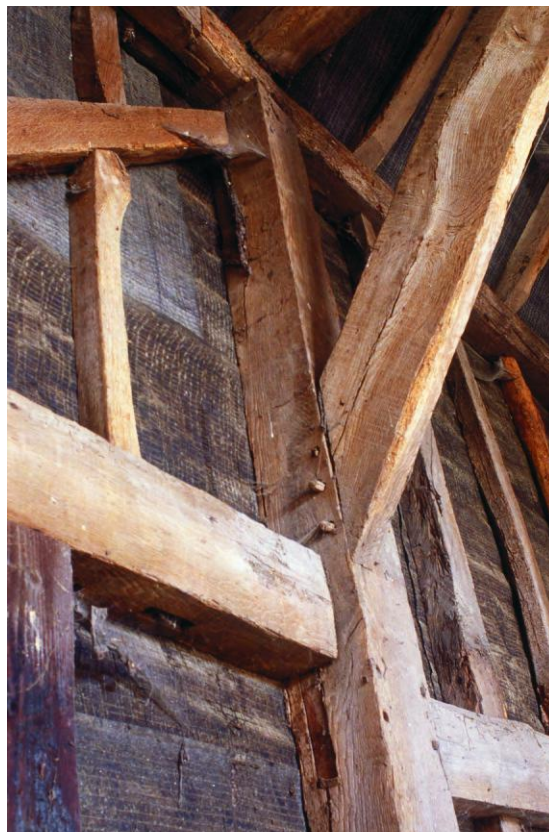
Fig 15 Detail of the raised midrail above the fireplace and the face-halved and bladed scarf joint in the wall plate
