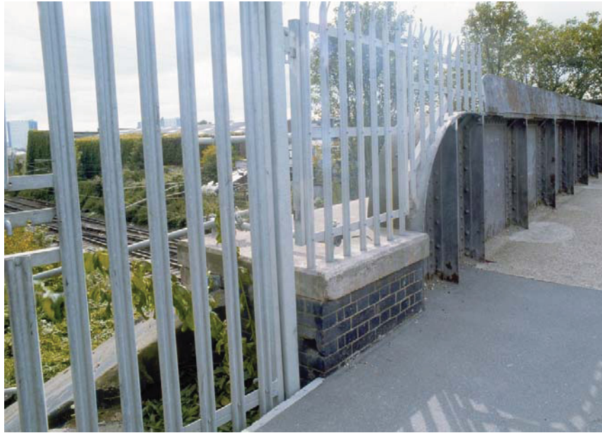
Plate 12 The east parapet wall and the altered bridge pier of The Waterden Road Bridge, looking south (34607010)
