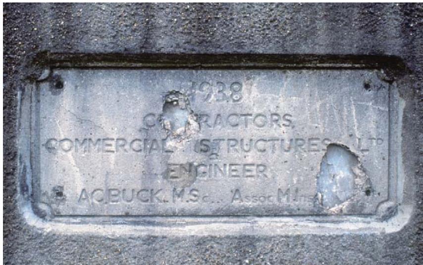
Plate 8 Damaged plaque on the north parapet wall of The Bridgewater Road Bridge, looking south (34707010)
