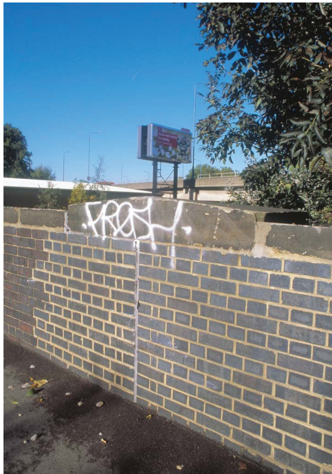
Plate 3 Detail of a repair to the north parapet wall of the Eastway Bridge, looking north-west (39507008)
