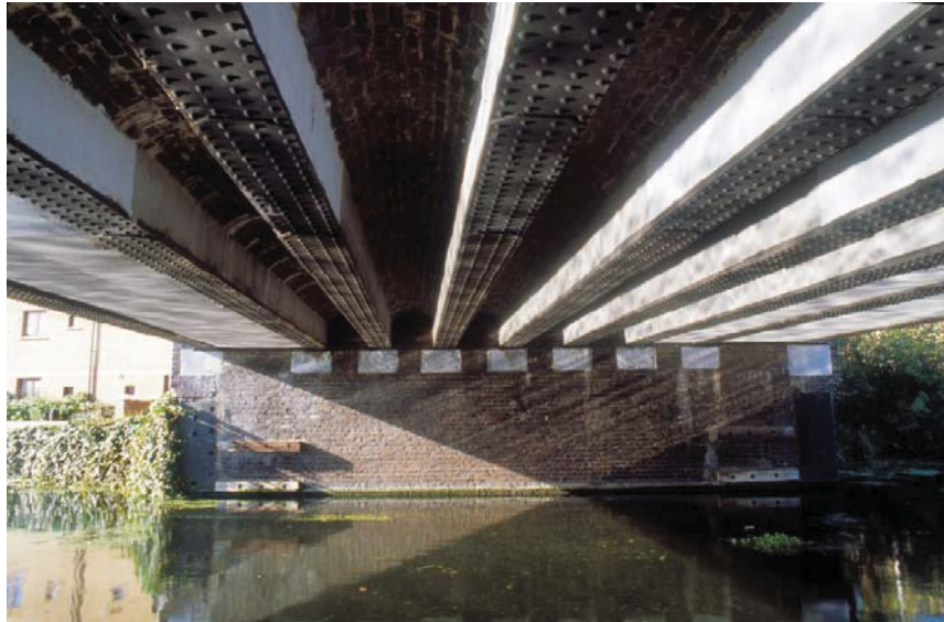
Plate 2 Riveted steel plate girders and brick jack arches of the Eastway Bridge, forming the bridge deck, looking west (39507016)
