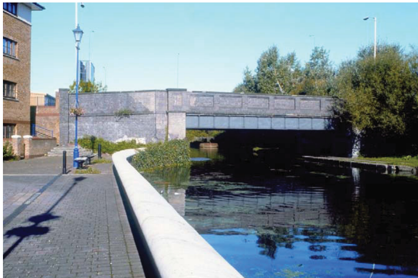
Plate 1 The south side of the Eastway Bridge seen from Meadow Close, looking north (39507013)
