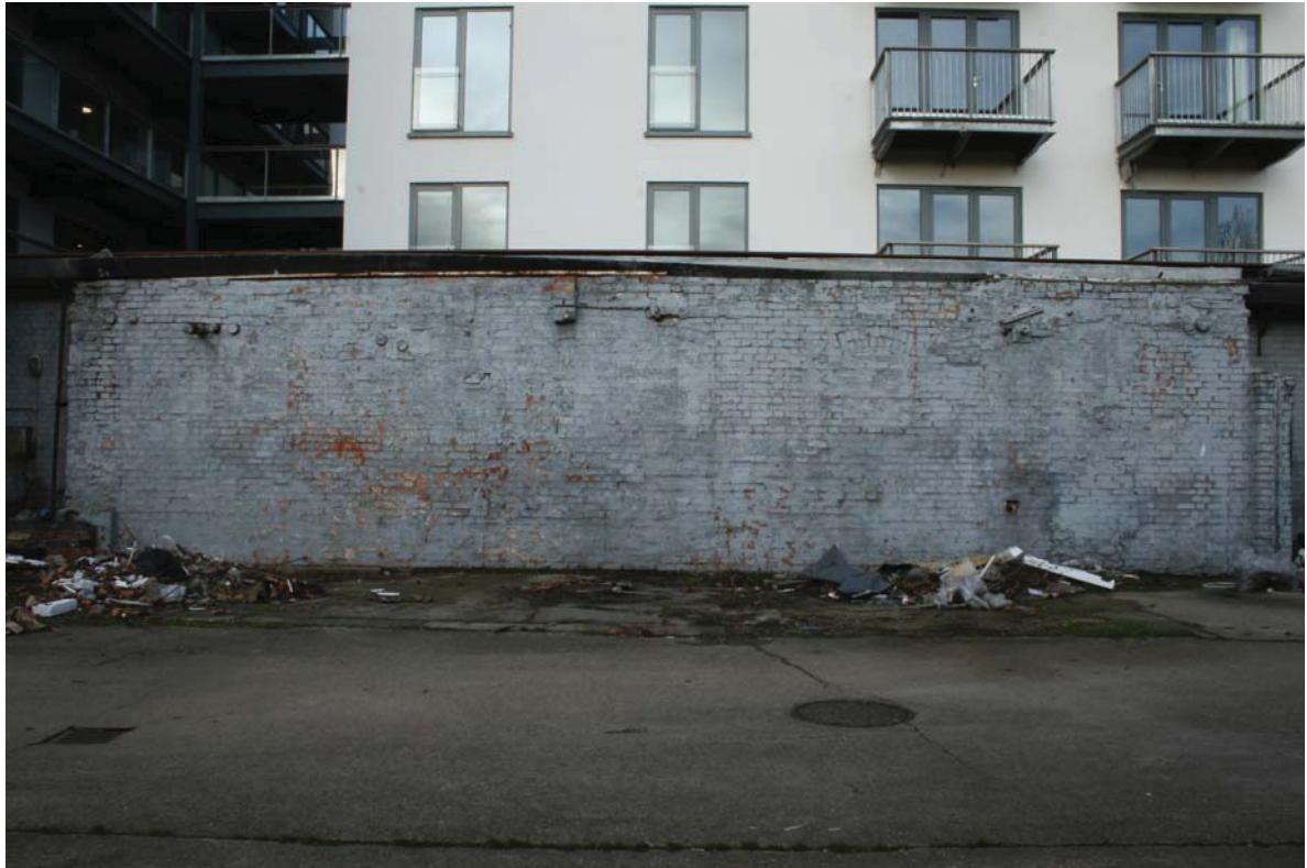
Plate 10 View looking N of the perimeter wall to the east of the Chimney (7)
