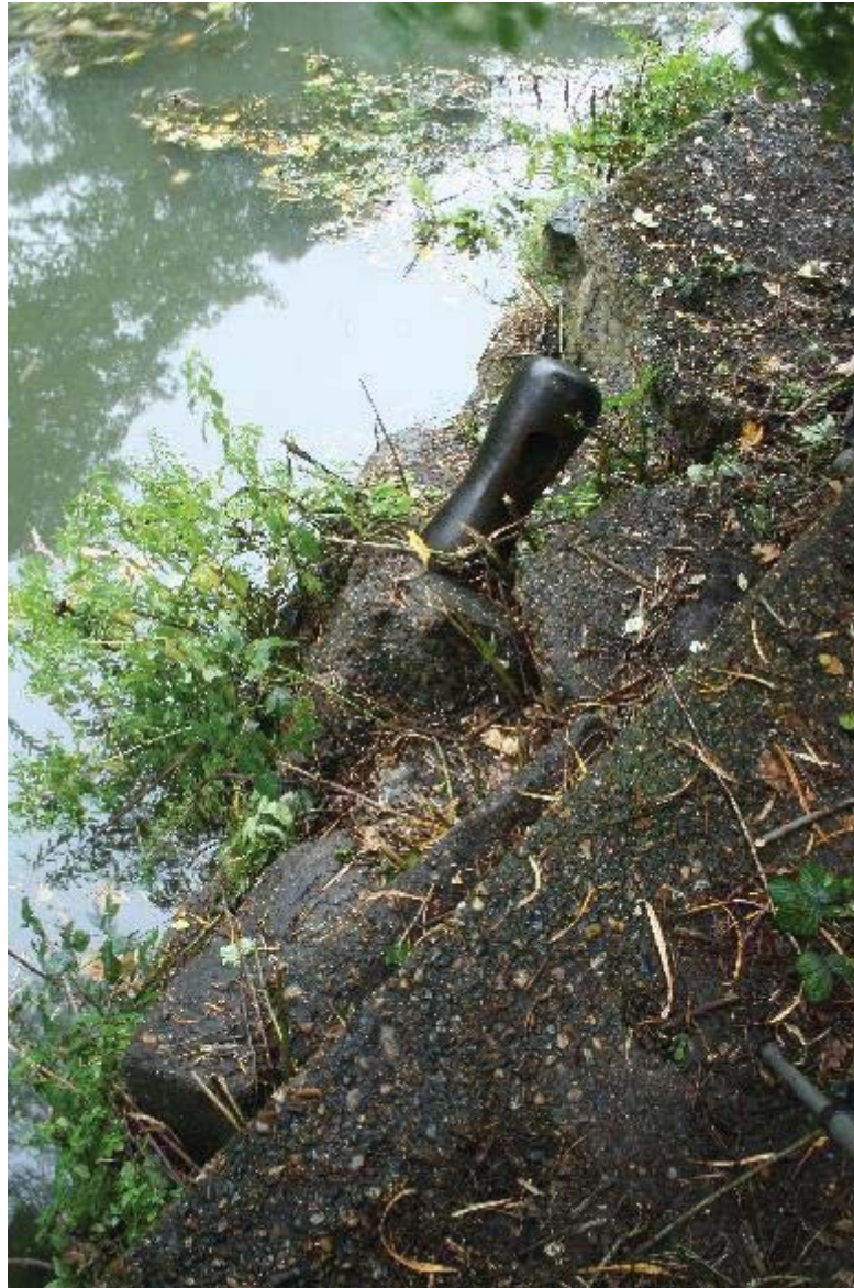
Plate 61 Detailed view of damaged eastern wing wall with metal mooring post, Pudding Mill River, looking north-northwest: OL-05407
