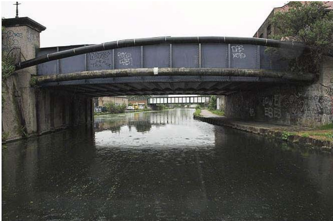
Plate 11 View of Eastway slip road bridge spanning the Lea Navigation, looking south: OL-01207
