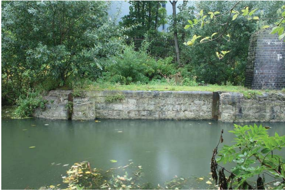
Plate 63 View of lock gate recess on east side of central island, Pudding Mill Lock, looking north-west: OL-05407
