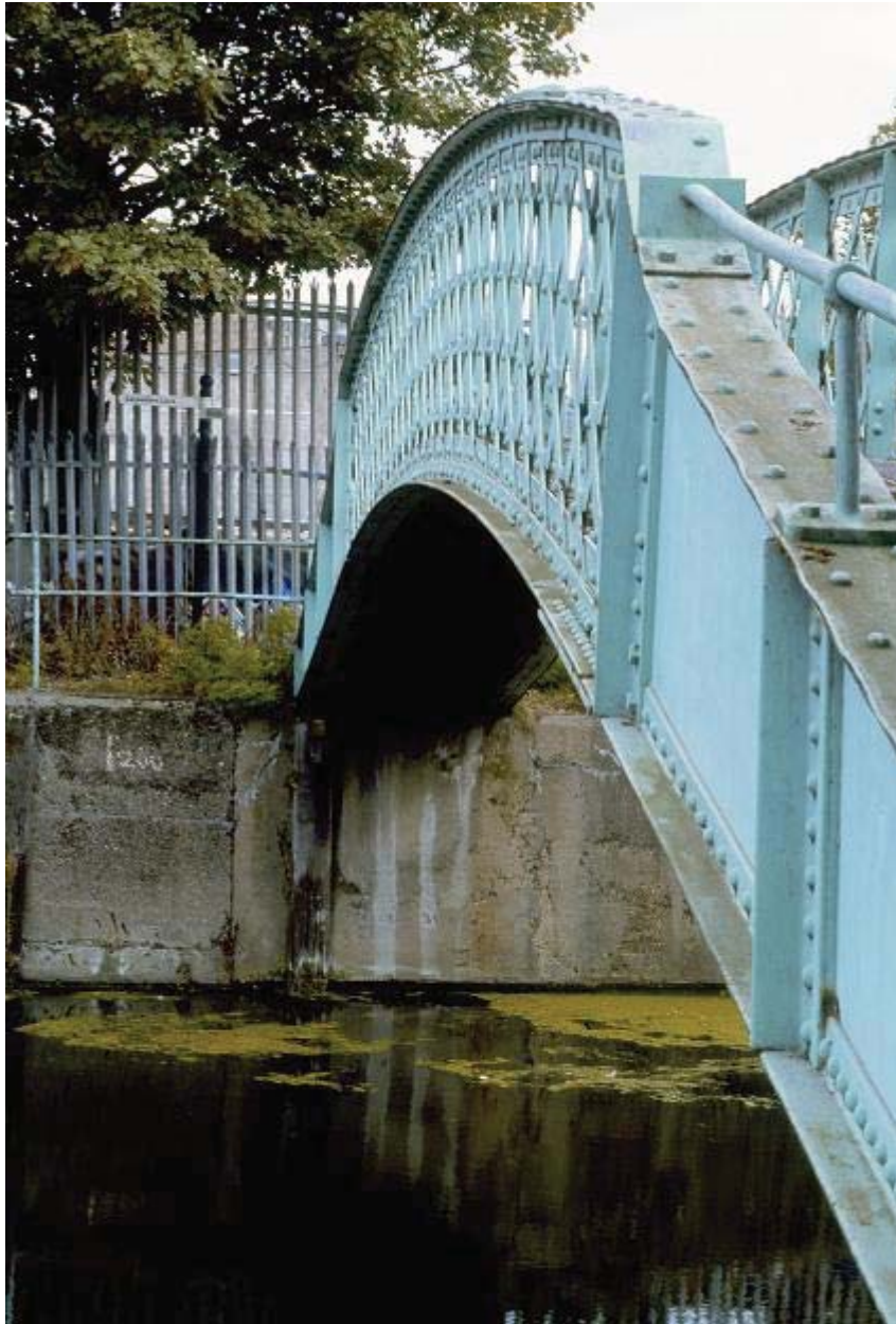
Plate 81 View of northern side of City Mill River Footbridge and anchorage in concrete wall, looking north-east: OL-03507
