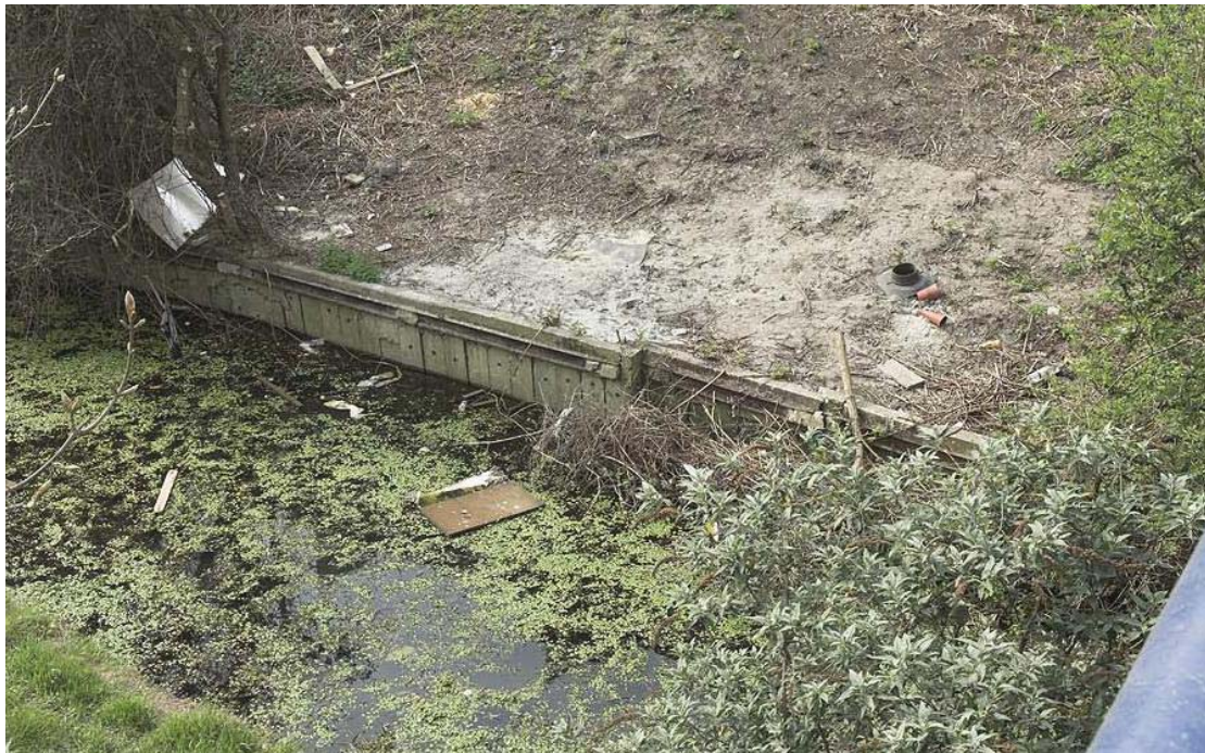
Plate 39 View of concrete platform and banking on Pudding Mill River, looking south-west: OL-01207
