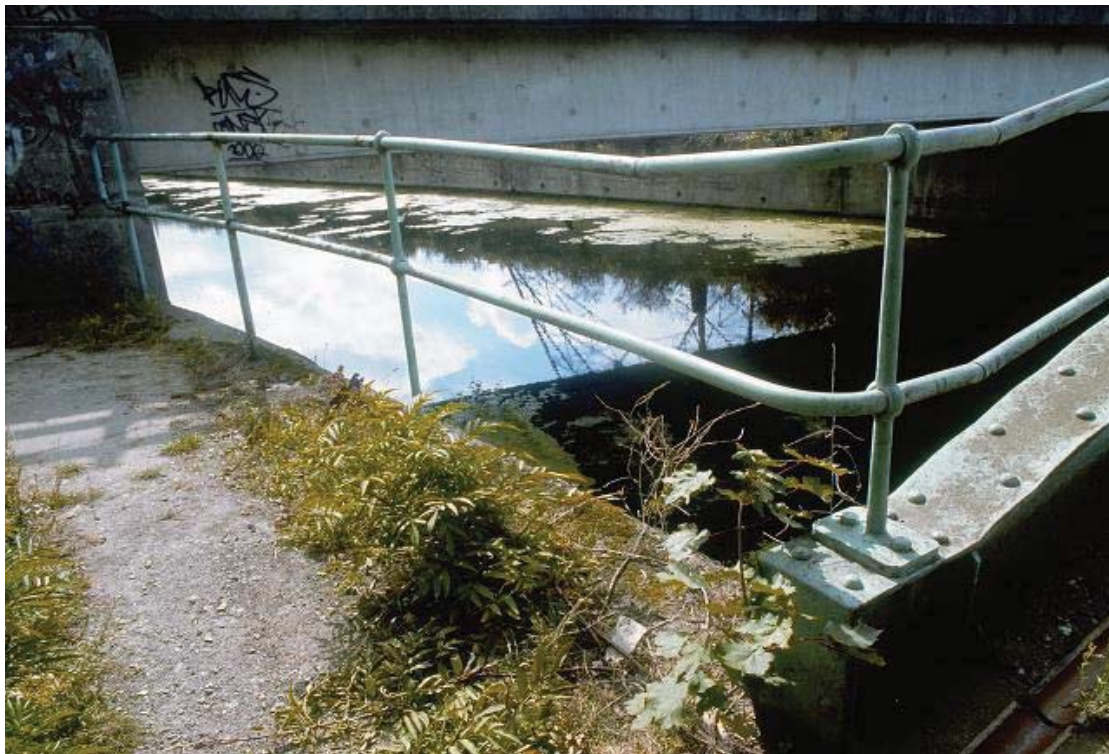
Plate 82 Detailed view of handrail at the south side of the eastern end of the City Mill River Footbridge, looking south: OL-03507
