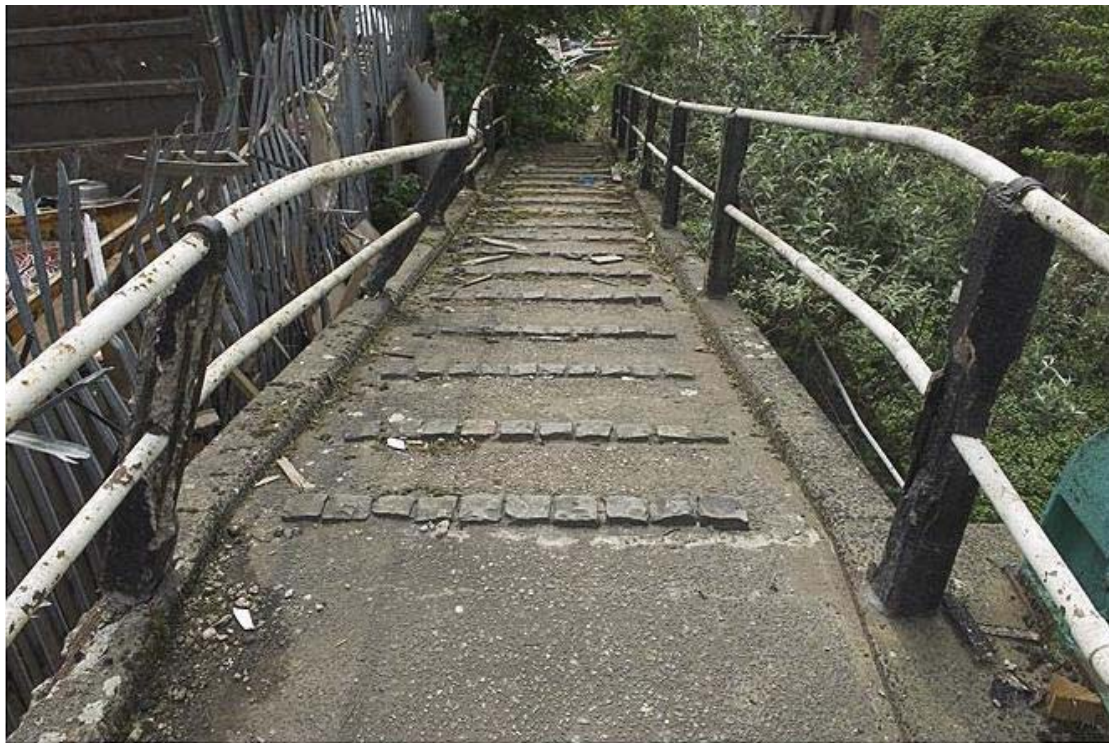
Plate 75 View of ramp with granite risers on the east bank of the River Lea, Carpenter's Lock, looking south-west: OL-03007
