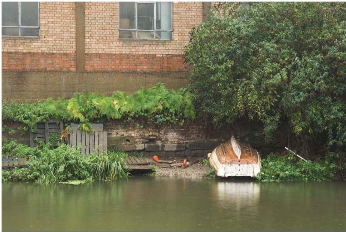
Plate 70 View of stone and brick riverbank wall showing building fabric, looking north-west: OL-07207
