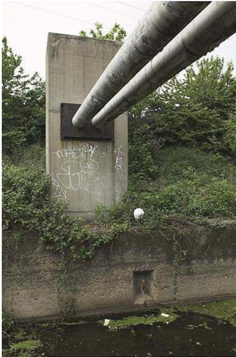
Plate 77 View of Thames Water sludge mains, immediately south of Carpenter's Lock, looking west: OL-03007
