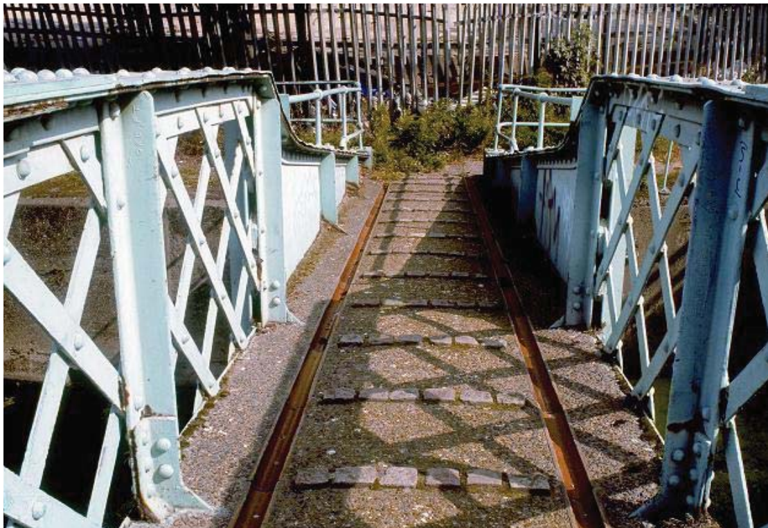
Plate 83 Detailed view showing granite set risers and inset open ceramic drainpipes, City Mill River Footbridge, looking north-east: OL-03507
