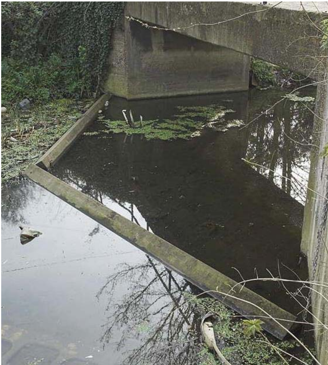
Plate 35 View of modern timber cofferdam on the Pudding Mill River, looking north- east: OL-01207
