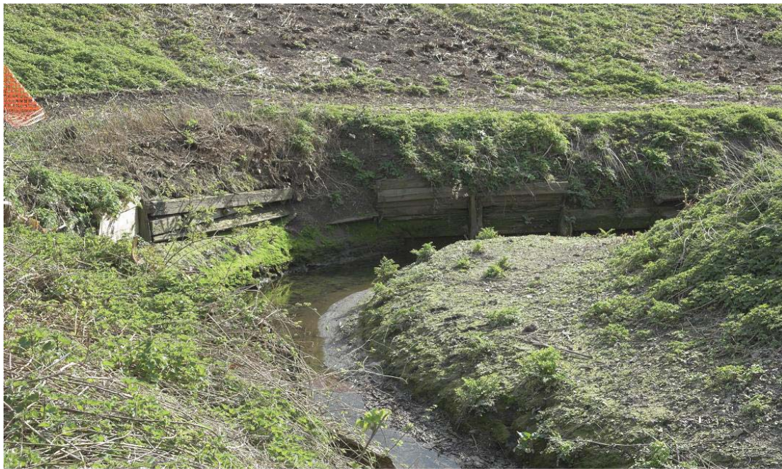
Plate 24 View of curve of Potter's Ditch with timber revetment, looking south-east: OL-02007
