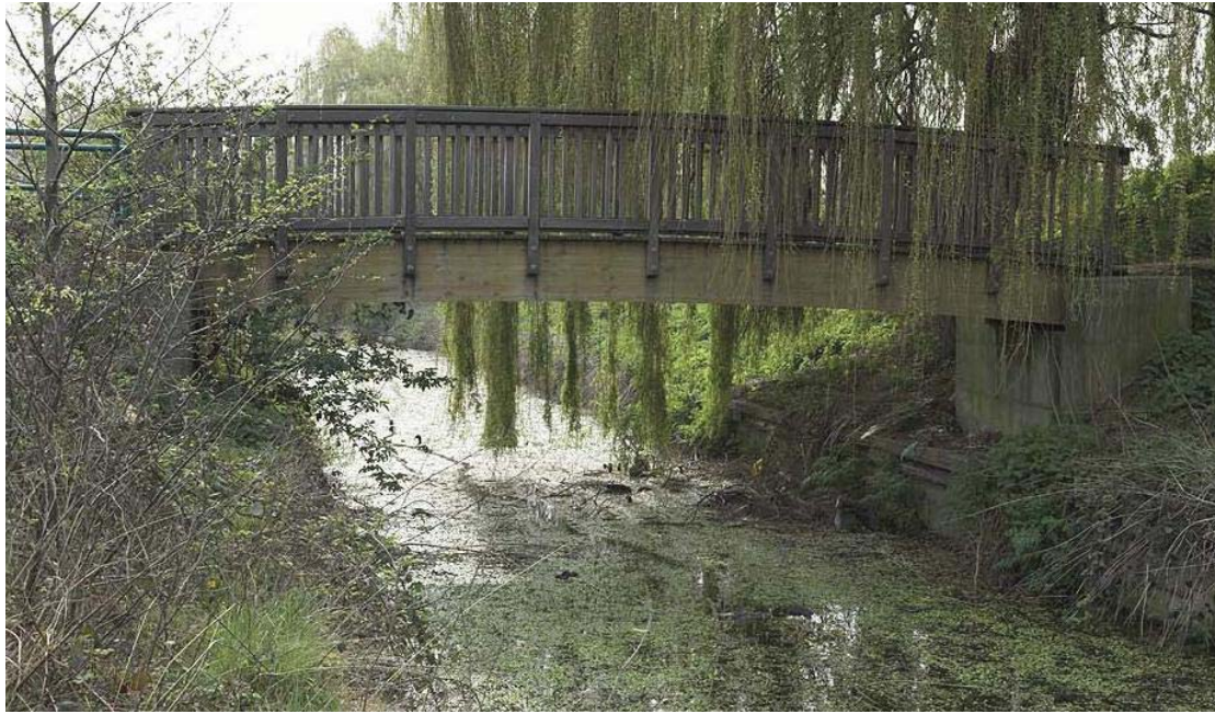
Plate 38 View of modern timber bridge spanning the Pudding Mill River, looking south-east: OL-01207
