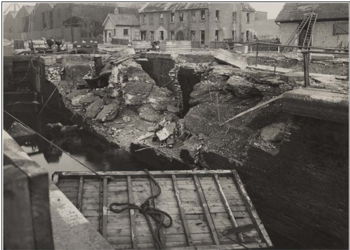
Plate 7 View of bomb damage to central pier at Old Ford Locks, October 1940 (LD PEM PS 159/0976, courtesy of Newham Local Studies and Archive Library): OL- 05007
