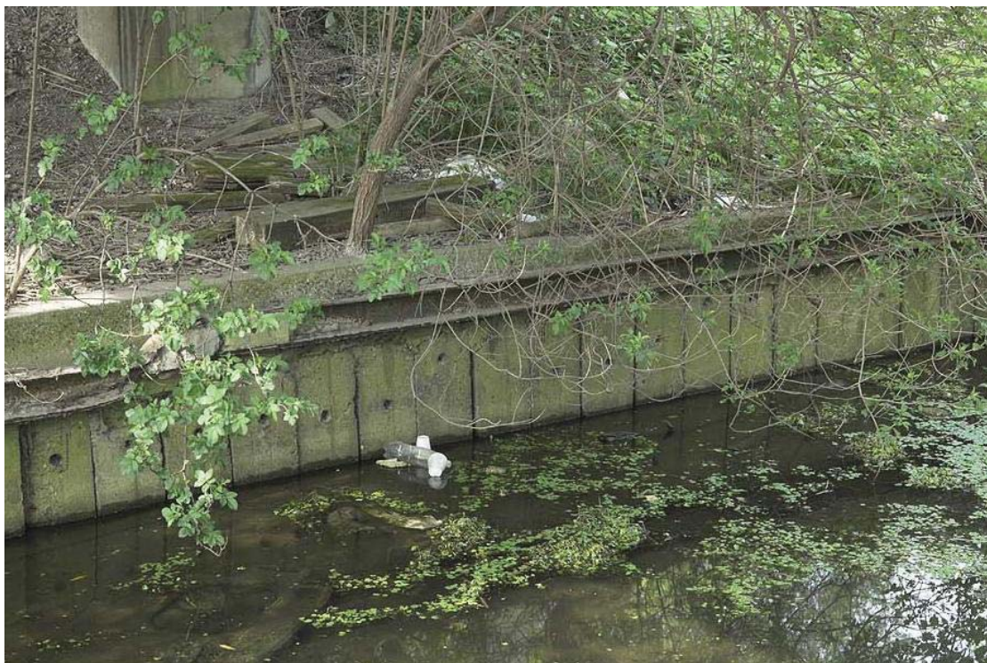
Plate 37 View of concrete pile west bank of Pudding Mill River, looking south-west: OL-01207
