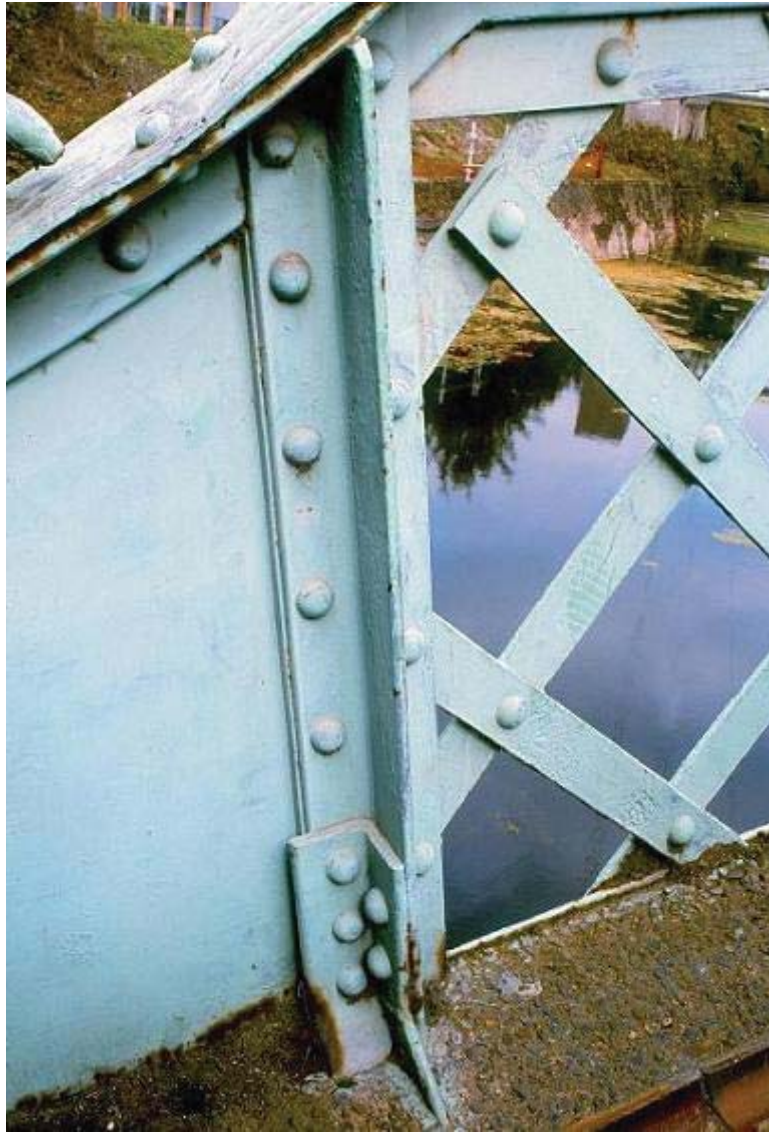
Plate 79 Detailed view of junction between steel panel and lattice on north side of City Mill River Footbridge, looking north: OL-03507
