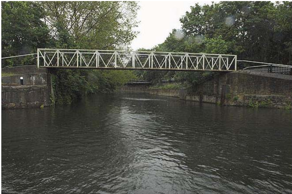
Plate 18 View of pedestrian bridge spanning the River Lea, south-east of Old Ford Locks, looking north-east: OL-01207
