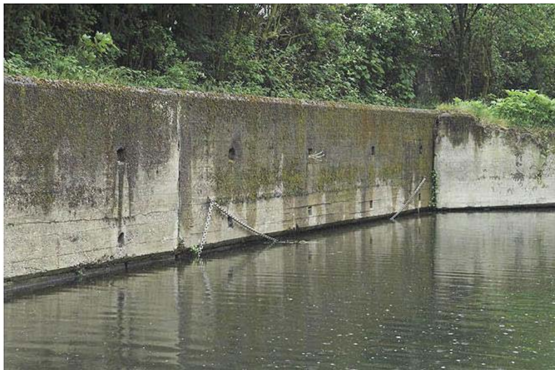
Plate 21 View of the east bank of the River Lea showing imprints of timber shuttering and sockets for mooring rings, looking south-west: OL-01207
