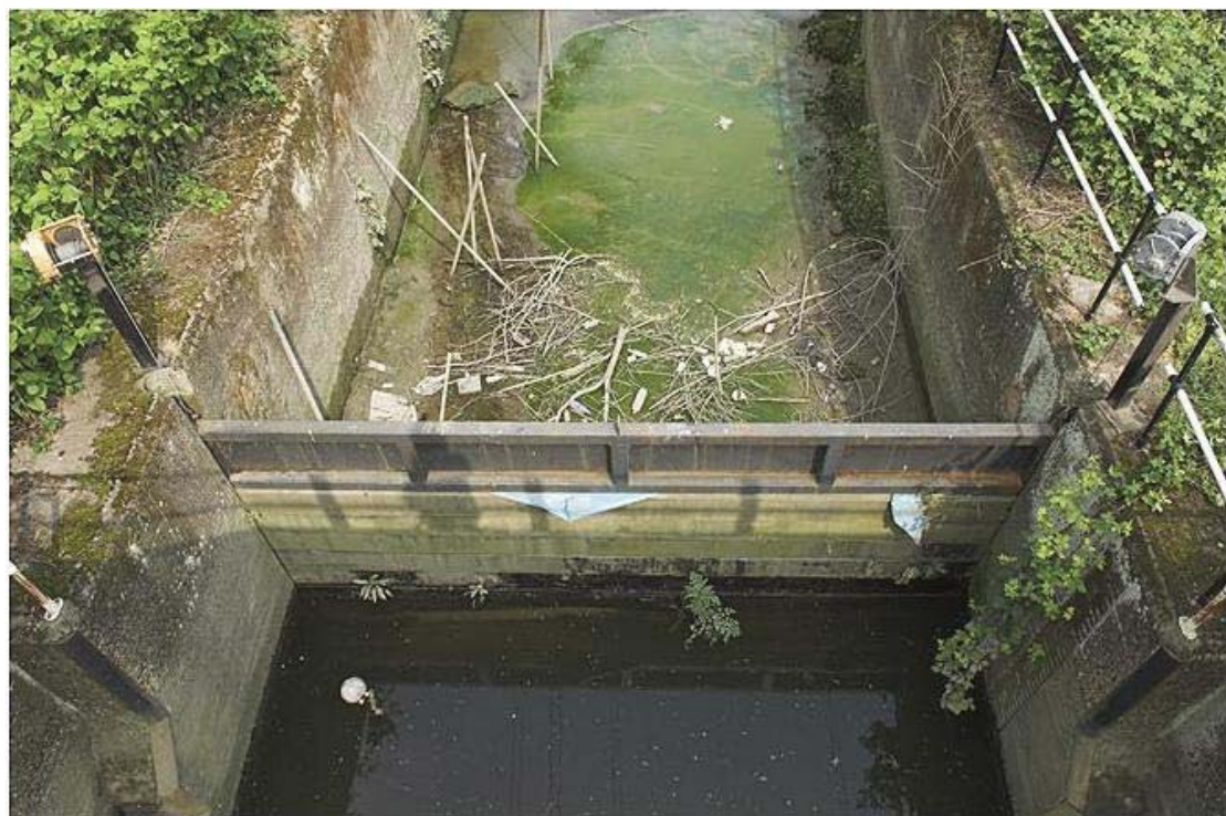
Plate 76 View of modern tide gate with associated machinery, Carpenter's Lock, looking north-east: OL-03007
