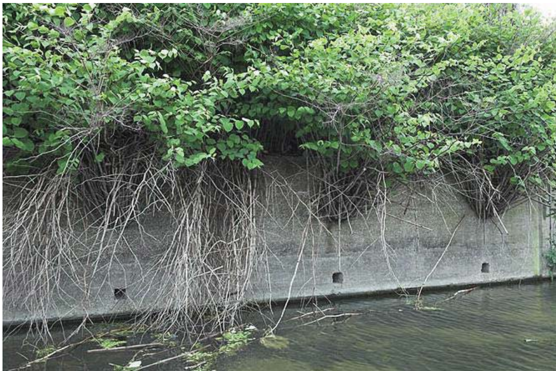
Plate 27 View of west bank of City Mill River with row of drainage holes immediately above waterline, looking west: OL-01207
