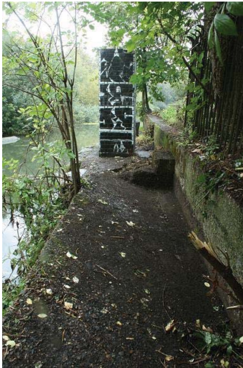
Plate 60 View of brick pier and east wing wall, Pudding Mill Lock, looking north: OL-05407
