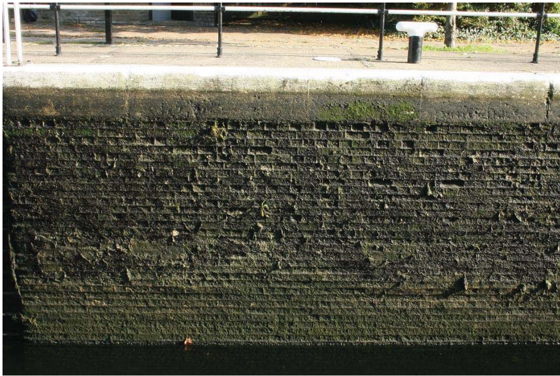
Plate 52 View of east wall in east chamber of Old Ford Locks, showing brick bond pattern, looking east: OL-05007
