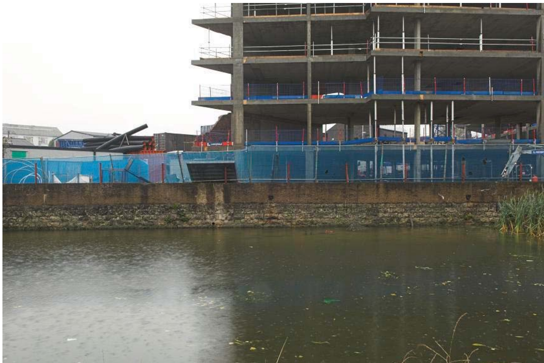
Plate 69 View of continuation of stone and brick riverbank wall, looking west- southwest: OL-07207
