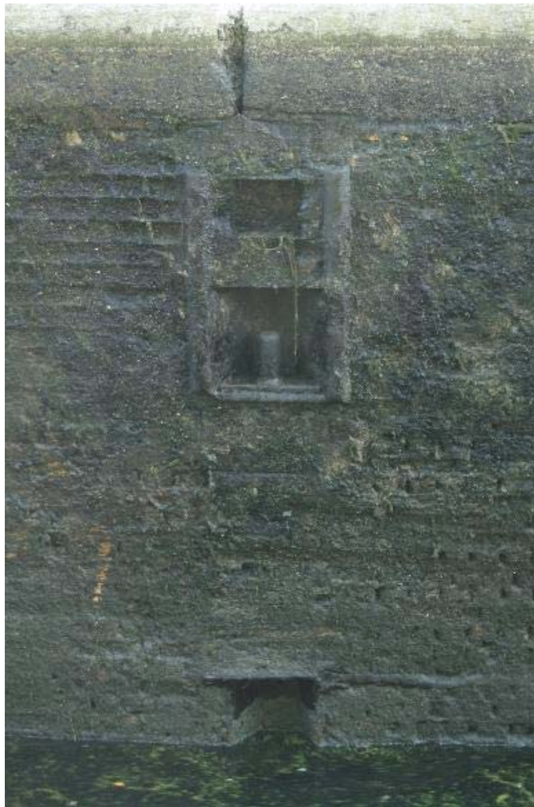
Plate 54 View of mooring hook set into east wall of east chamber, Old Ford Locks, looking east: OL-05007
