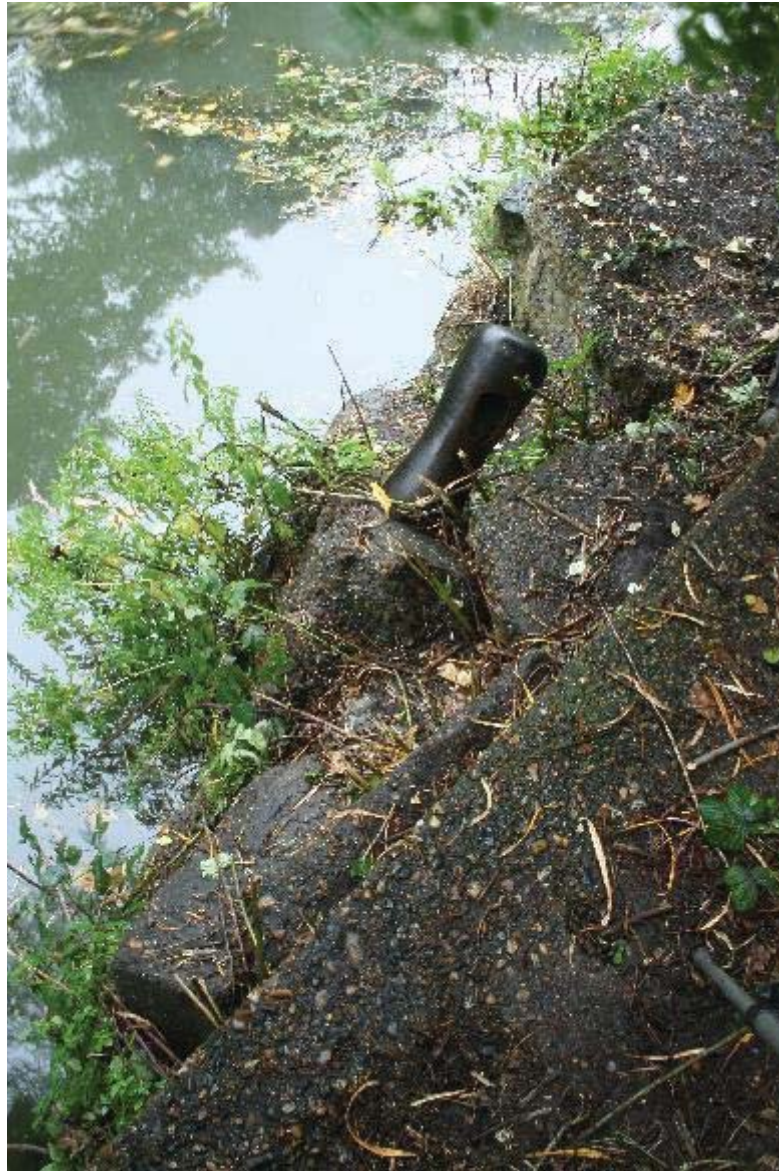
Plate 61 Detailed view of damaged eastern wing wall with metal mooring post, Pudding Mill River, looking north-northwest: OL-05407
