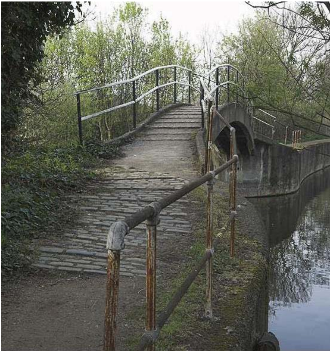
Plate 34 View of northern side of Pudding Mill River footbridge spanning the River Lea, looking south-west: OL-01207
