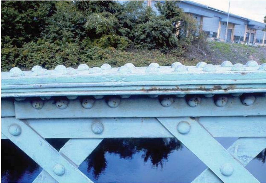
Plate 80 Detailed view of layered steel panels on northern side of City Mill River Footbridge, looking north-west: OL-03507
