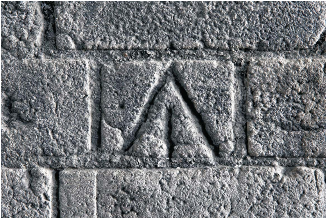
Plate 70 Detail of a benchmark carved into a brick at the northern end of the east abutment of the GER bridge over Carpenter's Road, looking north-east
