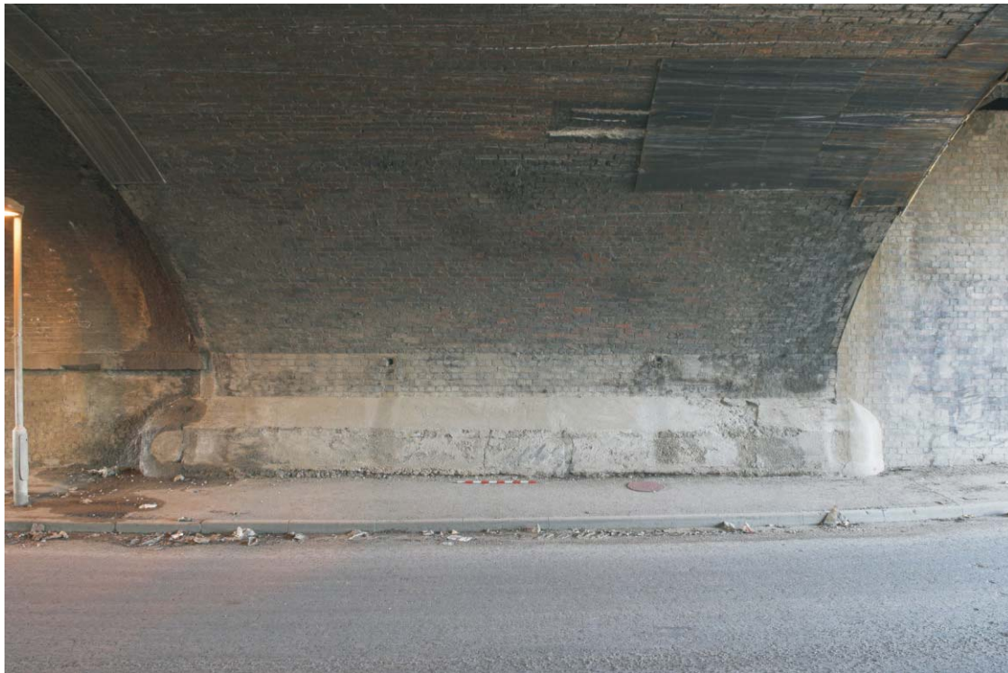
Plate 38 The northern end of the western abutment of the GER bridge across Pudding Mill Lane, looking south-west
