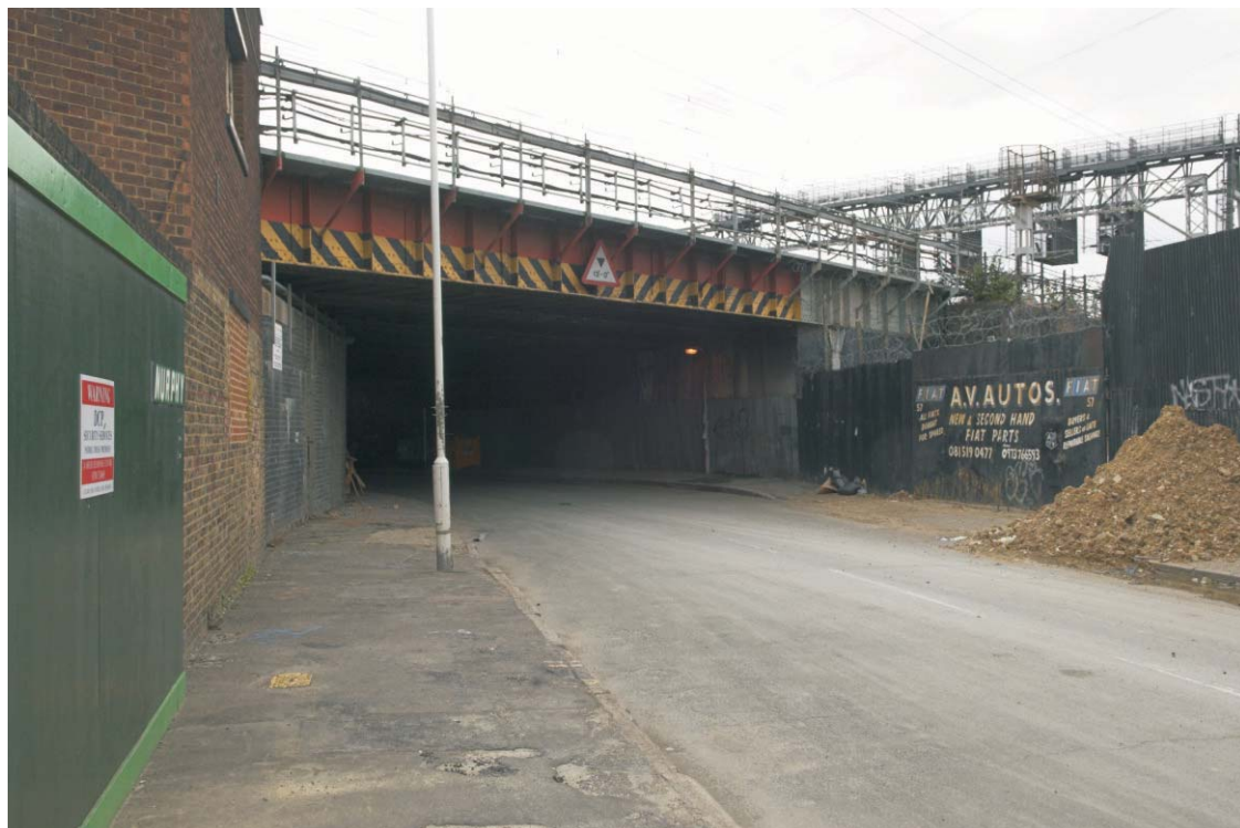
Plate 64 The northern side of the GER bridge over Warton Road, looking south-east
