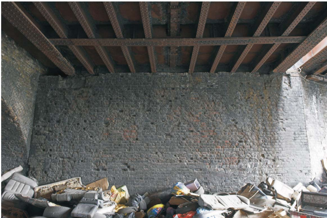
Plate 54 The northern end of the west abutment of the GER bridge over Marshgate Lane, looking south-west
