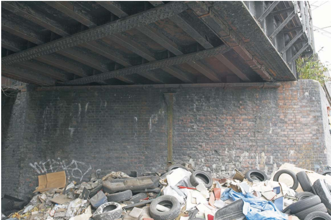
Plate 55 The northern end of the west abutment of the GER bridge over Marshgate Lane, looking south-west
