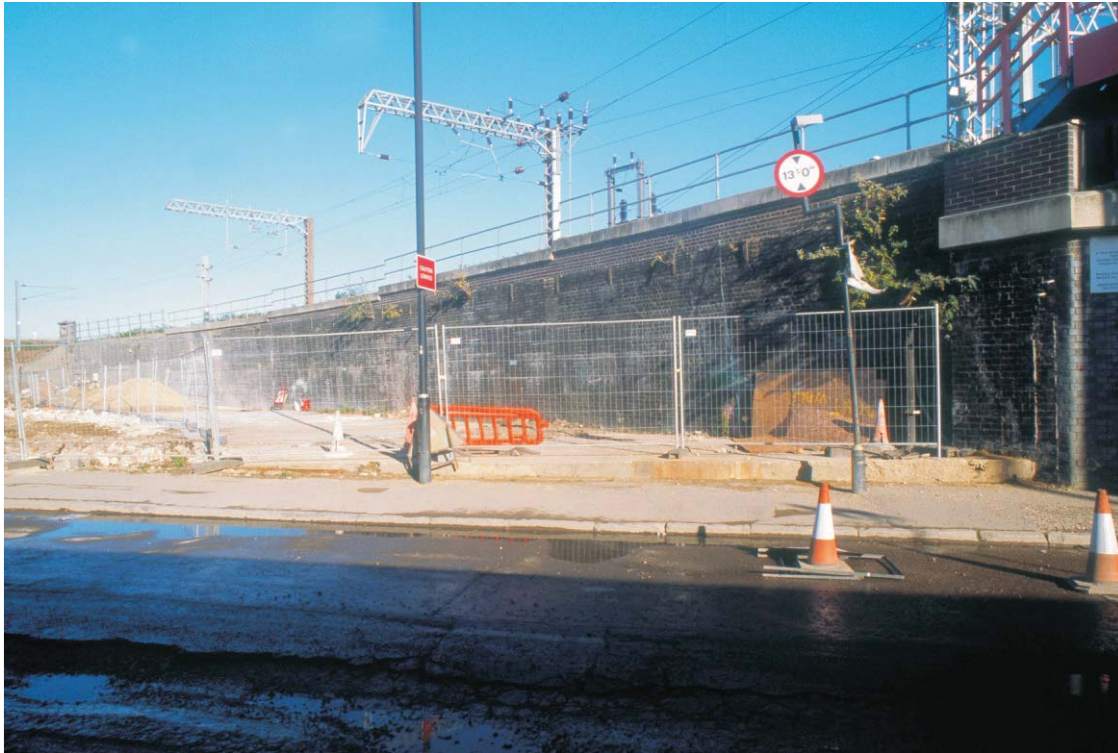
Plate 73 The brick retaining wall of the viaduct of the North London Line, looking north-east
