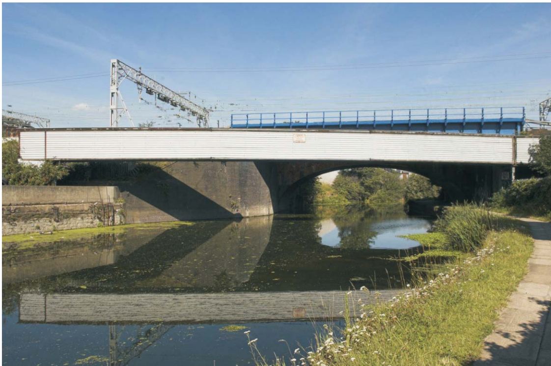
Plate 24 The southern side of the GER bridge over the River Lea, looking north-east
