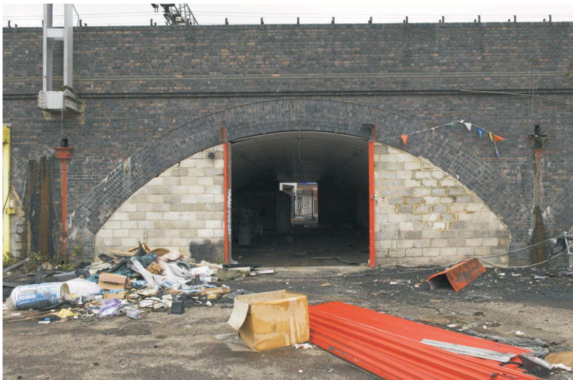
Plate 46 The exterior of the central arch of the Stratford viaduct, looking south-east
