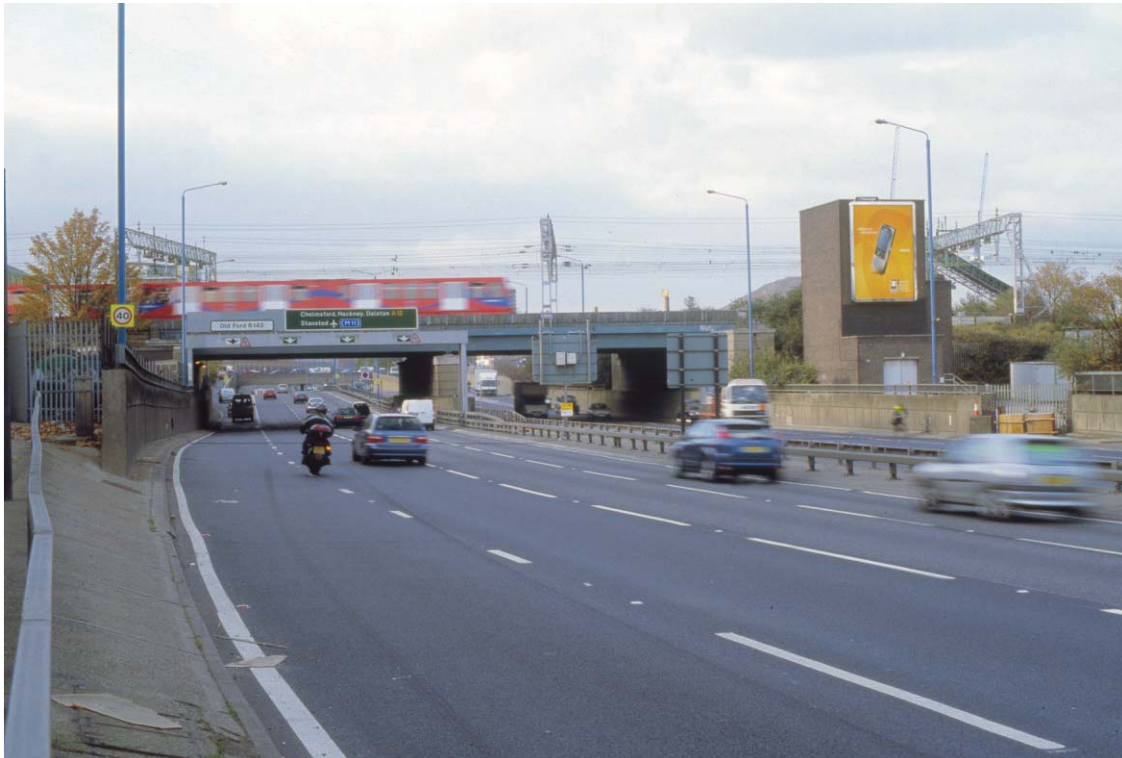
Plate 5 The GER bridge over the A12 Blackwall Tunnel Northern Approach, looking north
