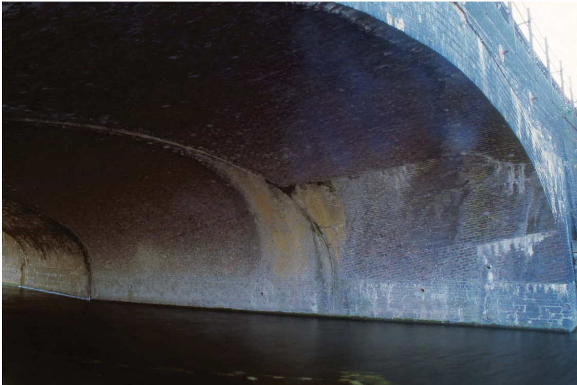
Plate 61 The northern end of the western abutment of the GER bridge over the City Mill River, looking south-west
