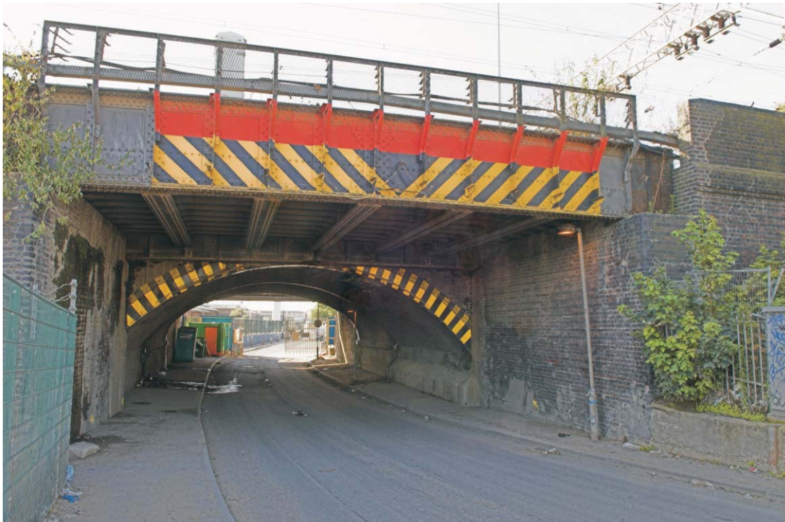
Plate 34 The northern side of the GER bridge across Pudding Mill Lane, looking south-east
