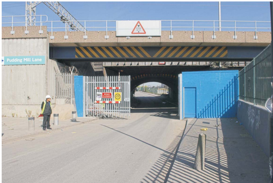
Plate 35 The southern side of the GER bridge across Pudding Mill Lane, looking north-west
