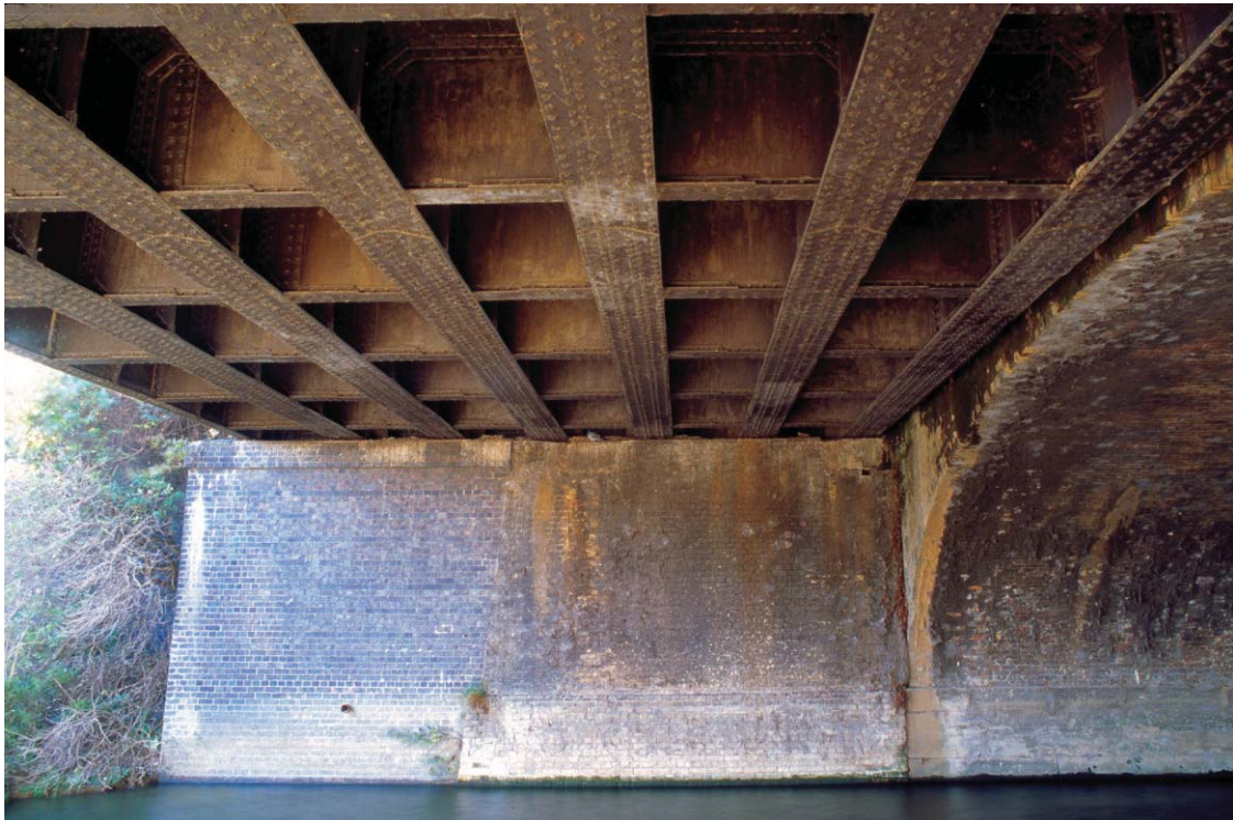
Plate 60 The southern end of the western abutment of the GER bridge over the City Mill River, looking south-west
