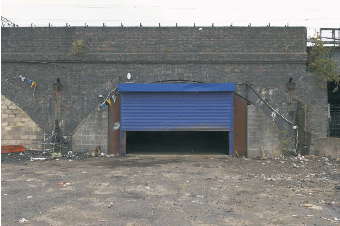
Plate 45 The exterior of the western arch of the Stratford viaduct, looking south-east
