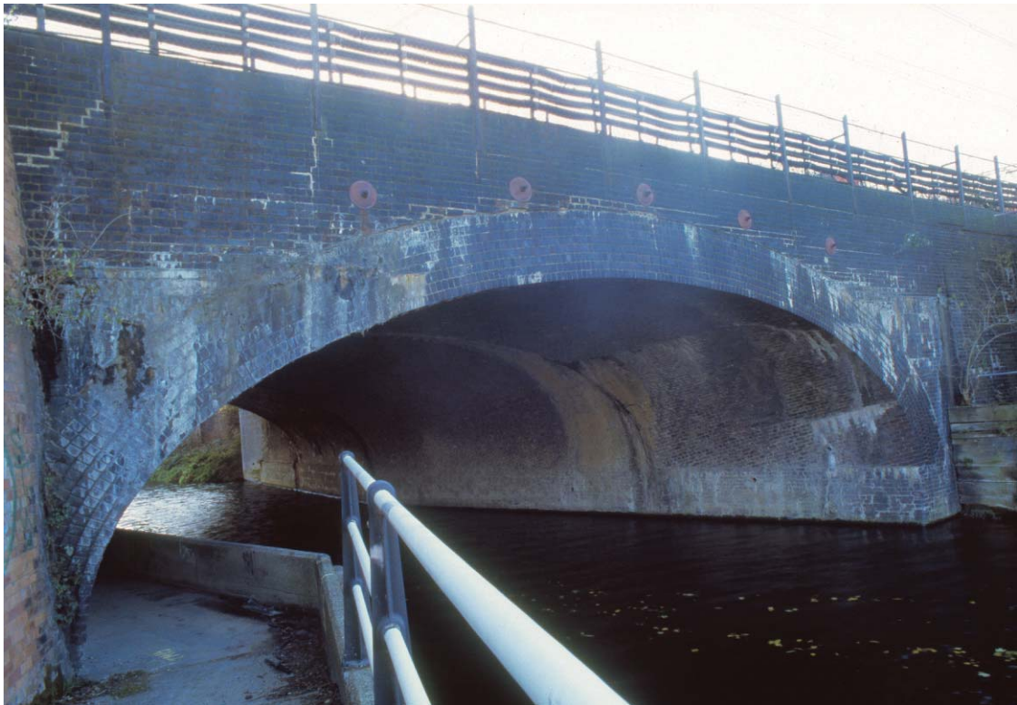
Plate 59 The northern side of the GER bridge over the City Mill River, looking south
