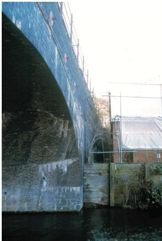
Plate 58 The northern side of the GER bridge over the City Mill River, looking south-west
