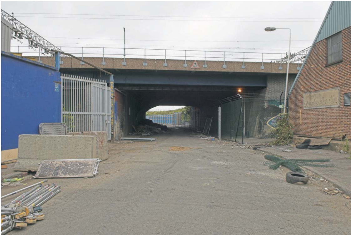
Plate 49 The southern side of the GER bridge over Marshgate Lane, looking north-west
