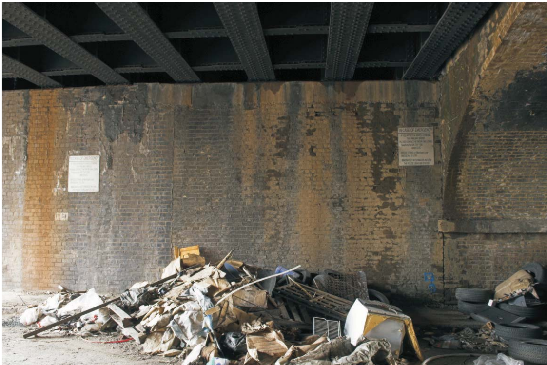
Plate 52 The southern end of the west abutment of the GER bridge over Marshgate Lane, looking south-west
