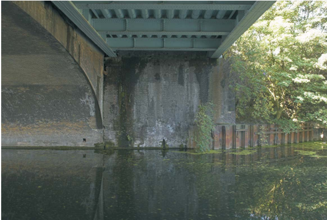
Plate 29 The northern end of the western abutment of the GER bridge over the River Lea, looking south-west
