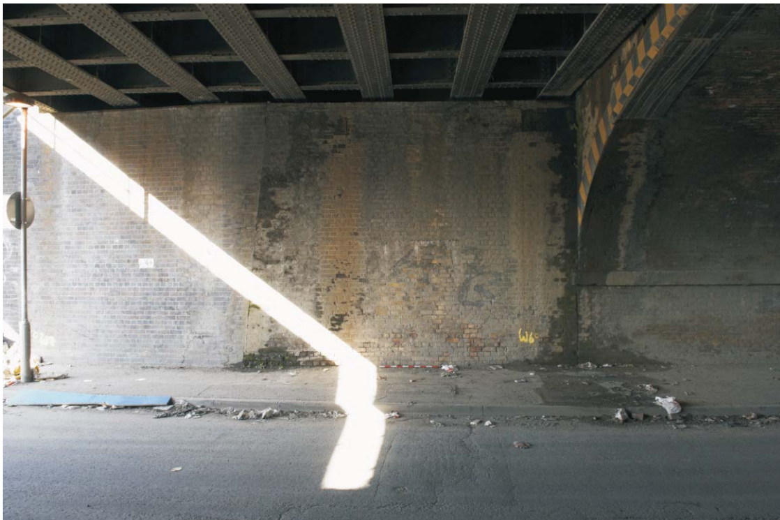
Plate 40 The southern end of the western abutment of the GER bridge across Pudding Mill Lane, looking south-west
