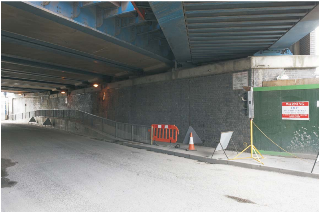
Plate 68 The northern end of the west abutment of the GER bridge over Carpenter's Road, looking south
