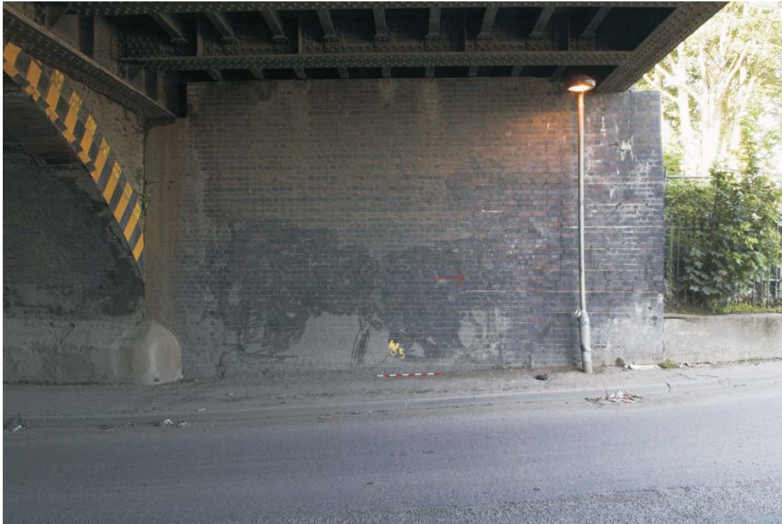
Plate 37 The northern end of the western abutment of the GER bridge across Pudding Mill Lane, looking south-west
