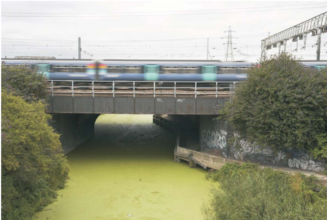
Plate 57 The southern side of the GER bridge over the City Mill River, looking north-west
