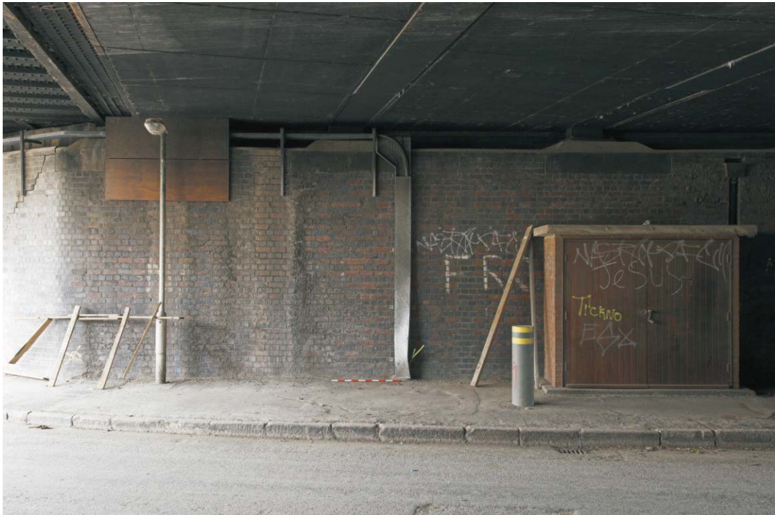
Plate 65 The northern end of the eastern abutment of the GER bridge over Warton Road, looking north-east
