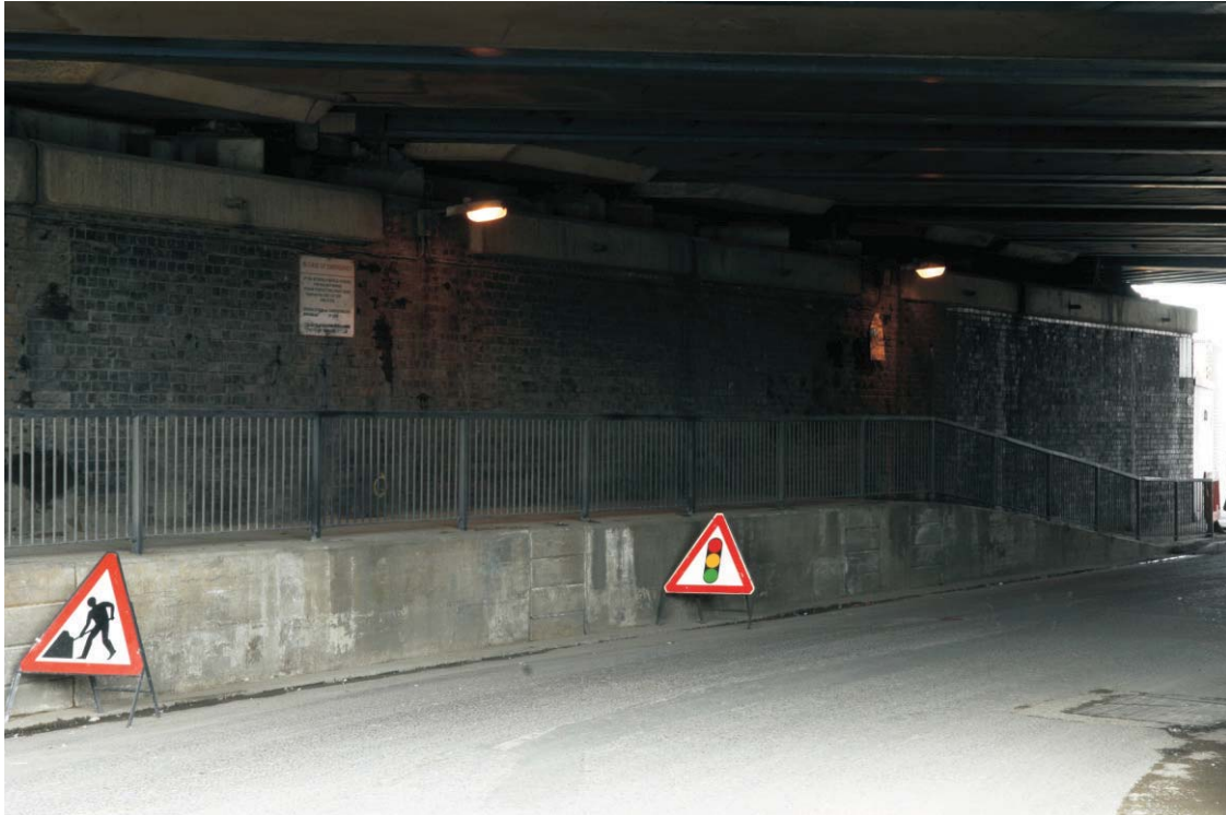
Plate 69 The northern end of the east abutment of the GER bridge over Carpenter's Road, looking south-east
