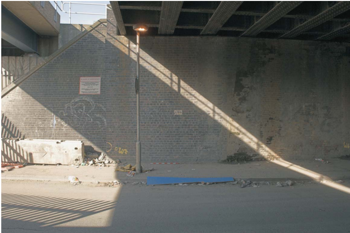
Plate 41 The southern end of the western abutment of the GER bridge across Pudding Mill Lane, looking south-west
