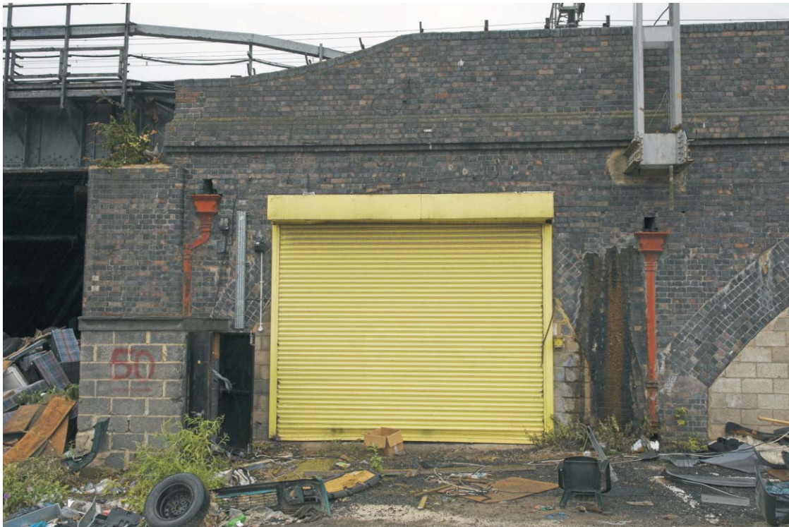
Plate 47 The exterior of the eastern arch of the Stratford viaduct, looking south-east
