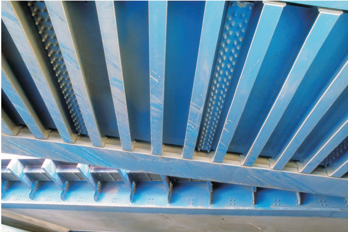
Plate 71 Detail of the steel decks on the northern side of the GER bridge over Carpenter's Road
