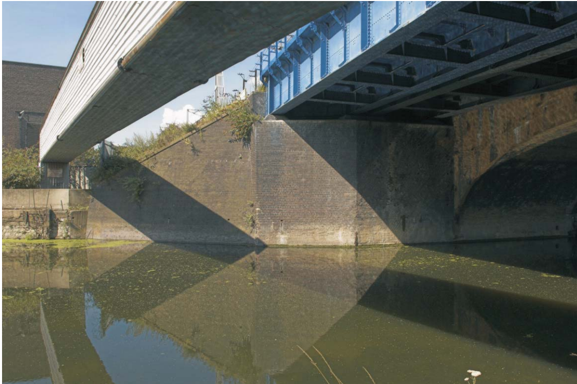
Plate 27 The southern end of the western abutment of the GER bridge over the River Lea, looking west
