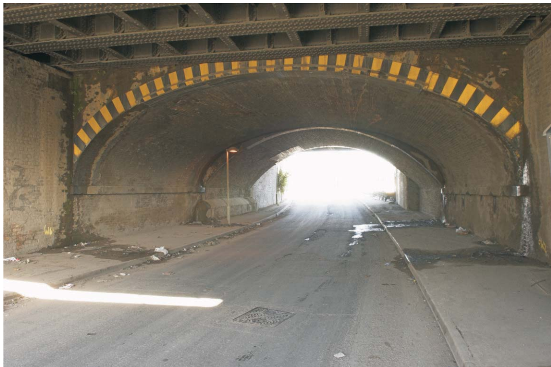
Plate 36 The elliptical Braithwaite arch of the primary phase of construction of the GER bridge over Pudding Mill Lane, looking north-west
