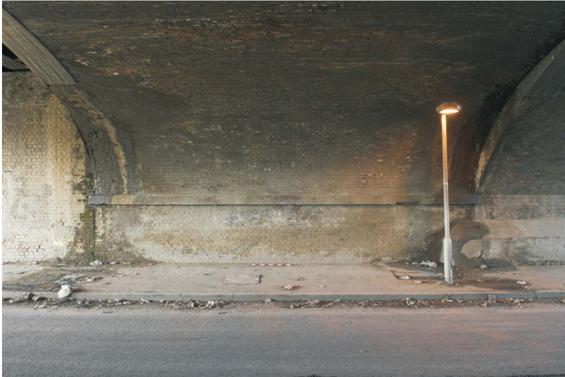
Plate 39 The centre of the western abutment of the GER bridge across Pudding Mill Lane, looking south-west
