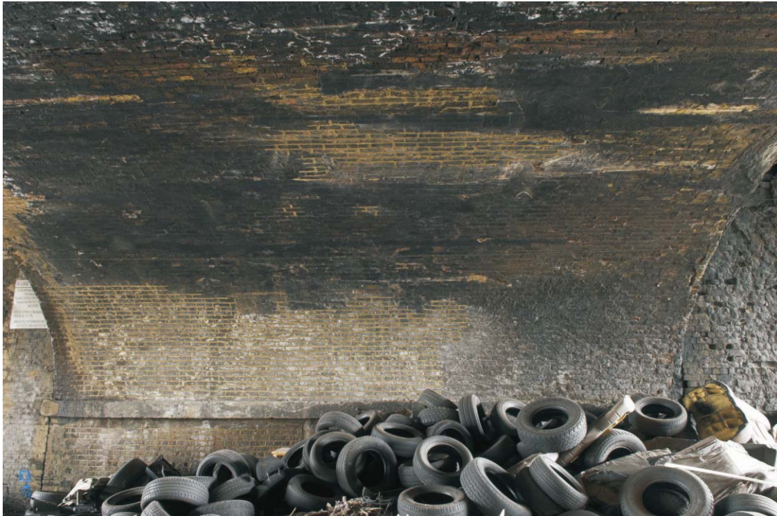
Plate 53 The centre of the west abutment of the GER bridge over Marshgate Lane, looking south-west
