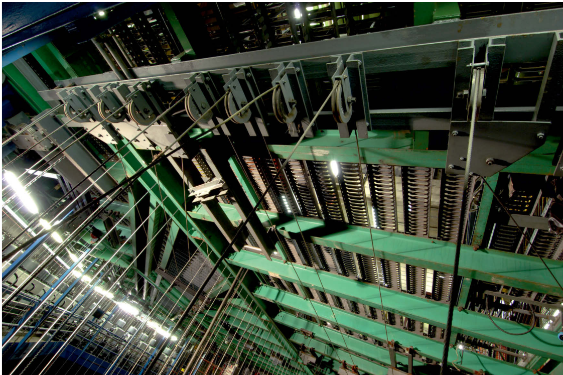
Fig 15 Looking up and to SW (ie toward downstage stage left), showing the counterweight loft block array suspended below the grid at the rear of the fly loft
