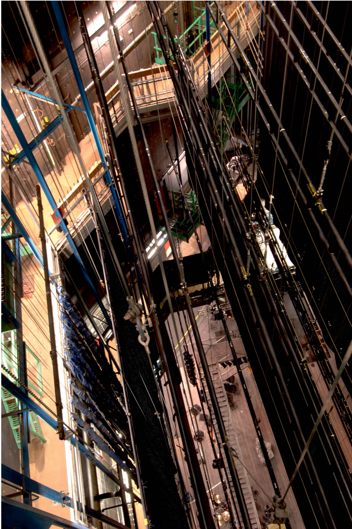
Fig 17 Looking down and to SE (ie upstage and toward the centre of stage right) from sub-grid level, showing the counterweight chains (wrapped in blue plastic) suspended in front of the galleries at the back of the fly loft (at left)
