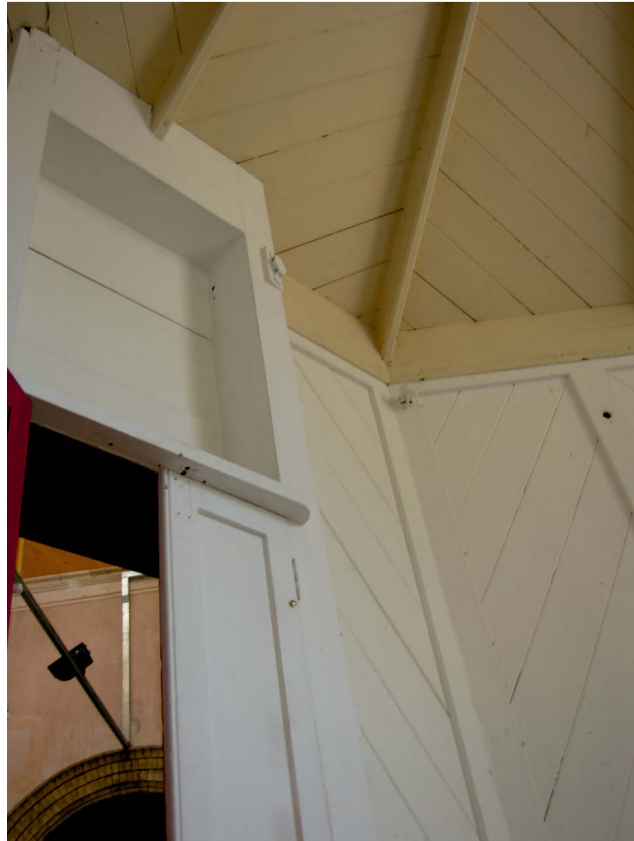
Fig 36 Task 18, detail of pulleys around ticket hatch in south east wall of ticket office, looking south east
