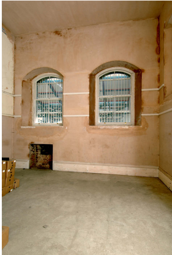
Fig 44 Task 25, the east room of the south tower, looking east, showing the two windows and a fireplace beneath
