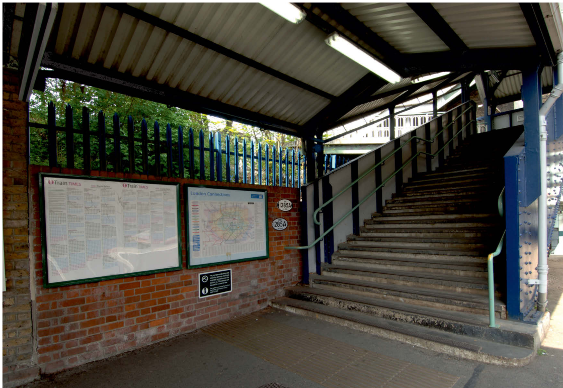
Fig 29 Task 11, brick wall, tactile paving and metal fence, Platform 1, looking south west
