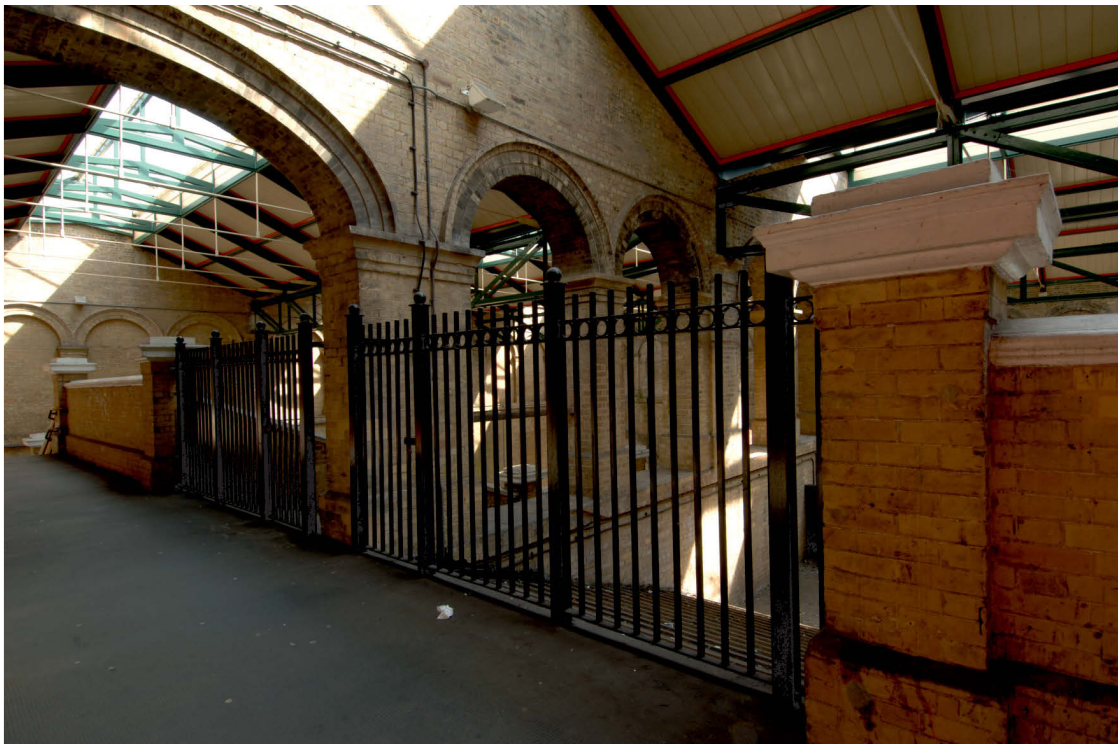
Fig 31 Task 13 railings at the head of former stairs to island platform looking north east
