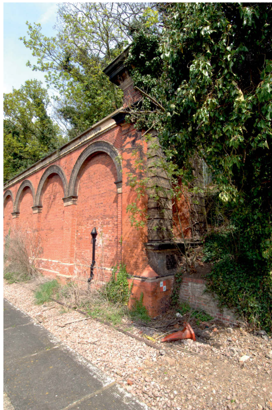
Fig 27 Task 9 detail of the buttress at the east end of the wall on Platform 4, looking north west
