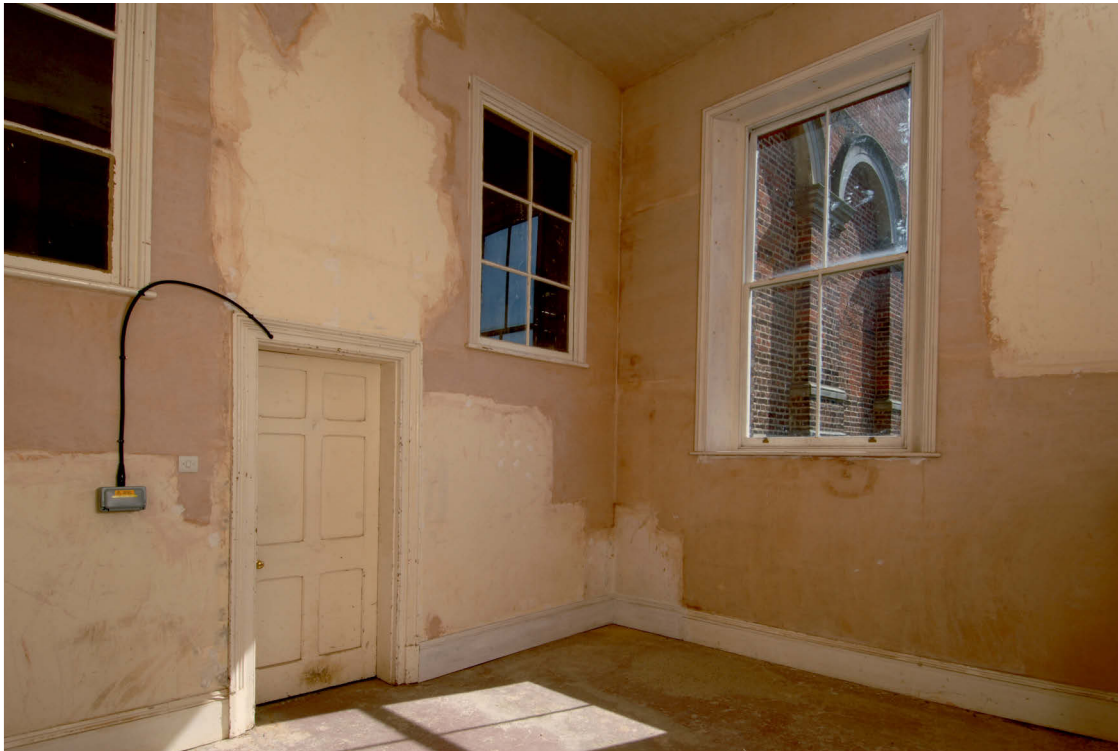
Fig 22 Task 5 internal view of the window to the south in east wall of south tower, looking north east. (will remain in revised plan)
