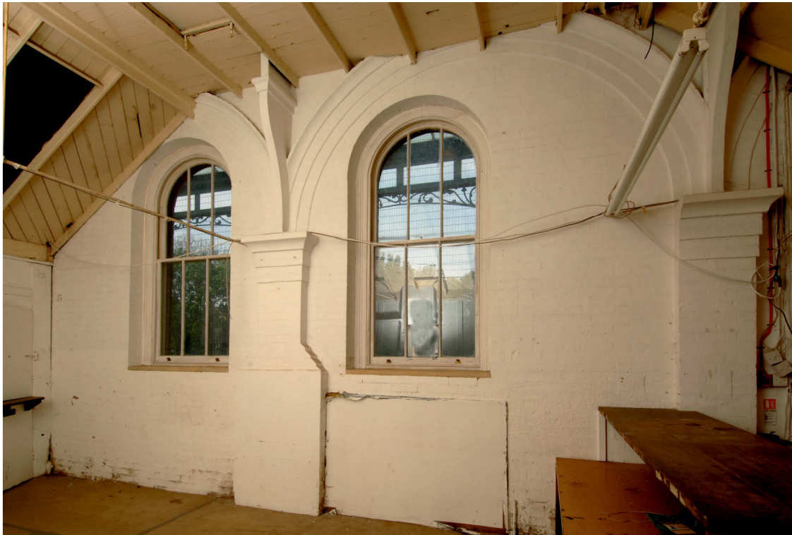
Fig 38 Task 18, internal west wall of ticket hall building and chimney breast within ticket office, looking west
