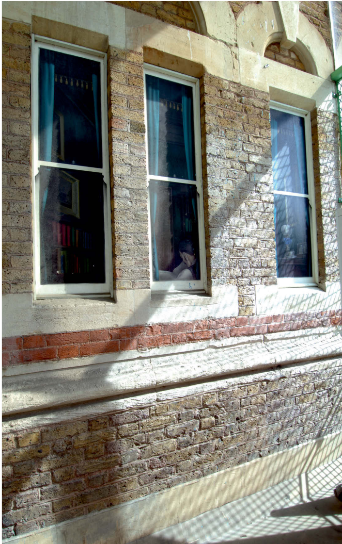
Fig 20 Task 4 south external wall of the south tower looking north, within the entrance hall showing boarded and painted windows
