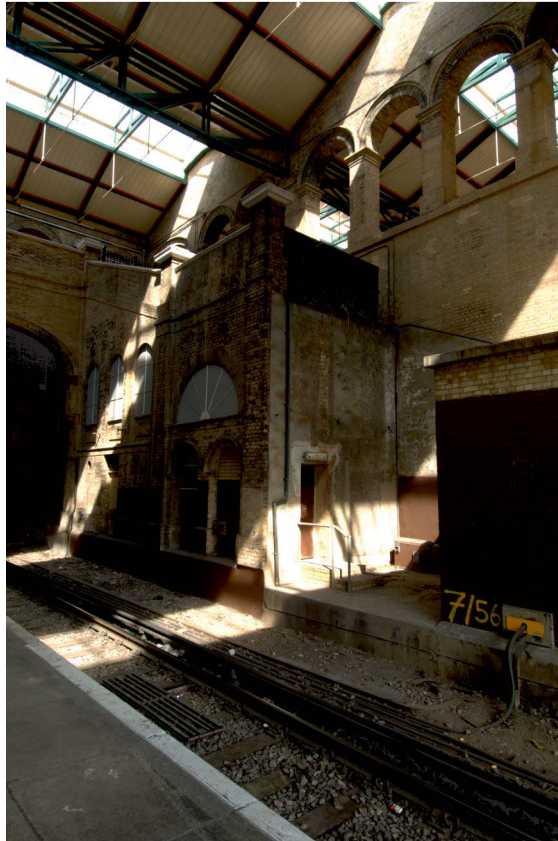
Fig 28 Task 10, stairs down to east side of island platform , main building, looking north west
