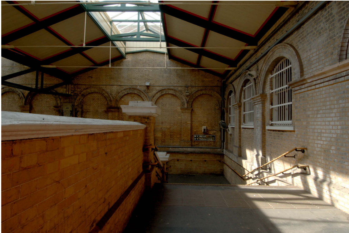
Fig 48 Task 28 wall at ticket hall level on the landing between Platforms 3 and 4, looking south
