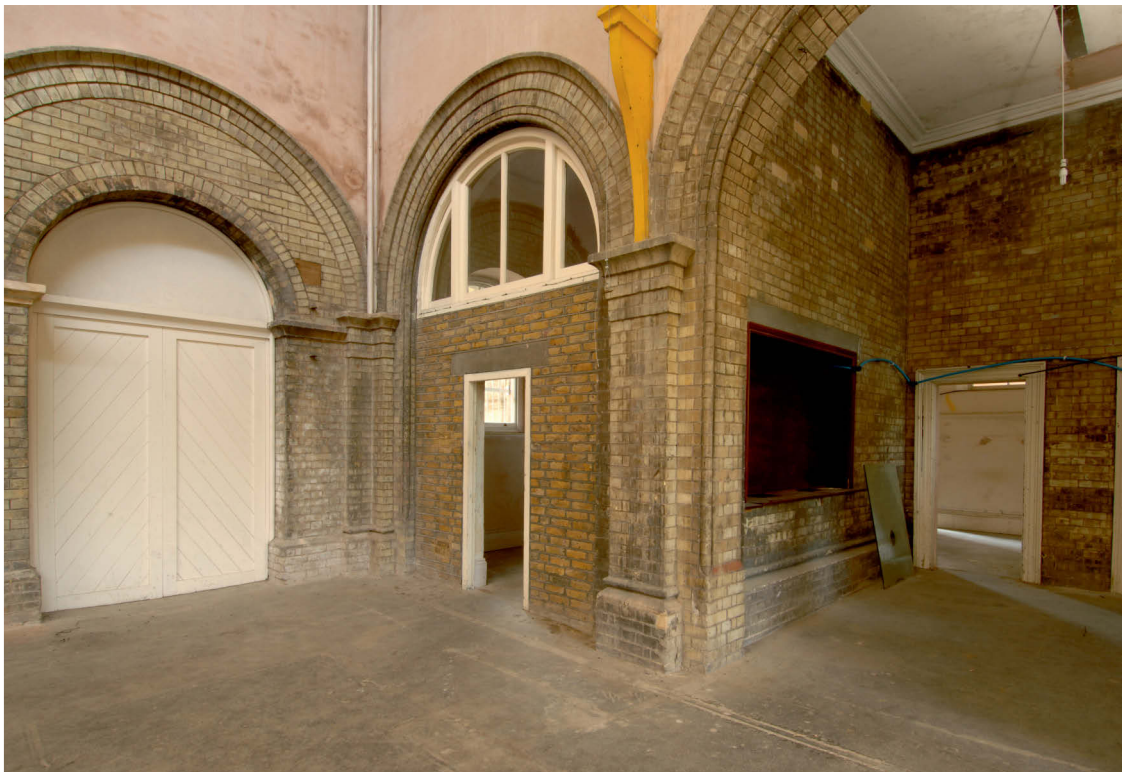
Fig 39 Tasks 19 and 21, bricked up arch in south east corner of the ticket hall, looking south east and the west facing side wall with ticket desk Task 21
