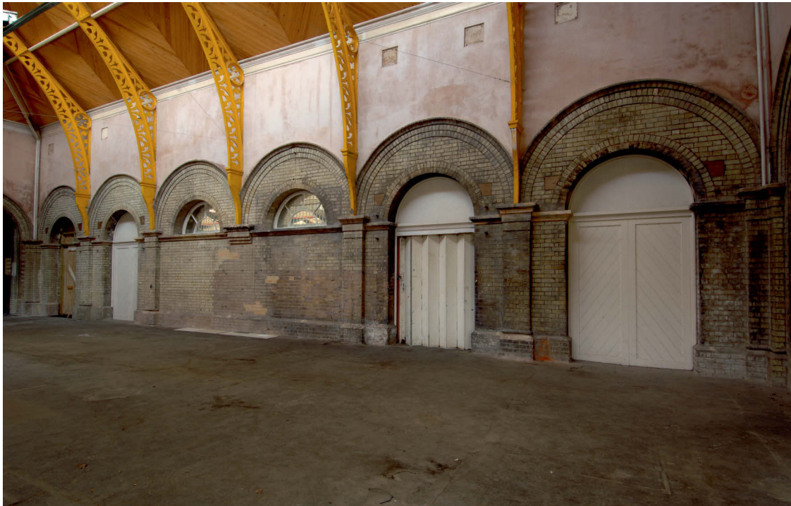
Fig 32 Tasks 14, 15 16 and 17 internal view of doorways from ticket hall to Platforms 3 and 4, looking north east
