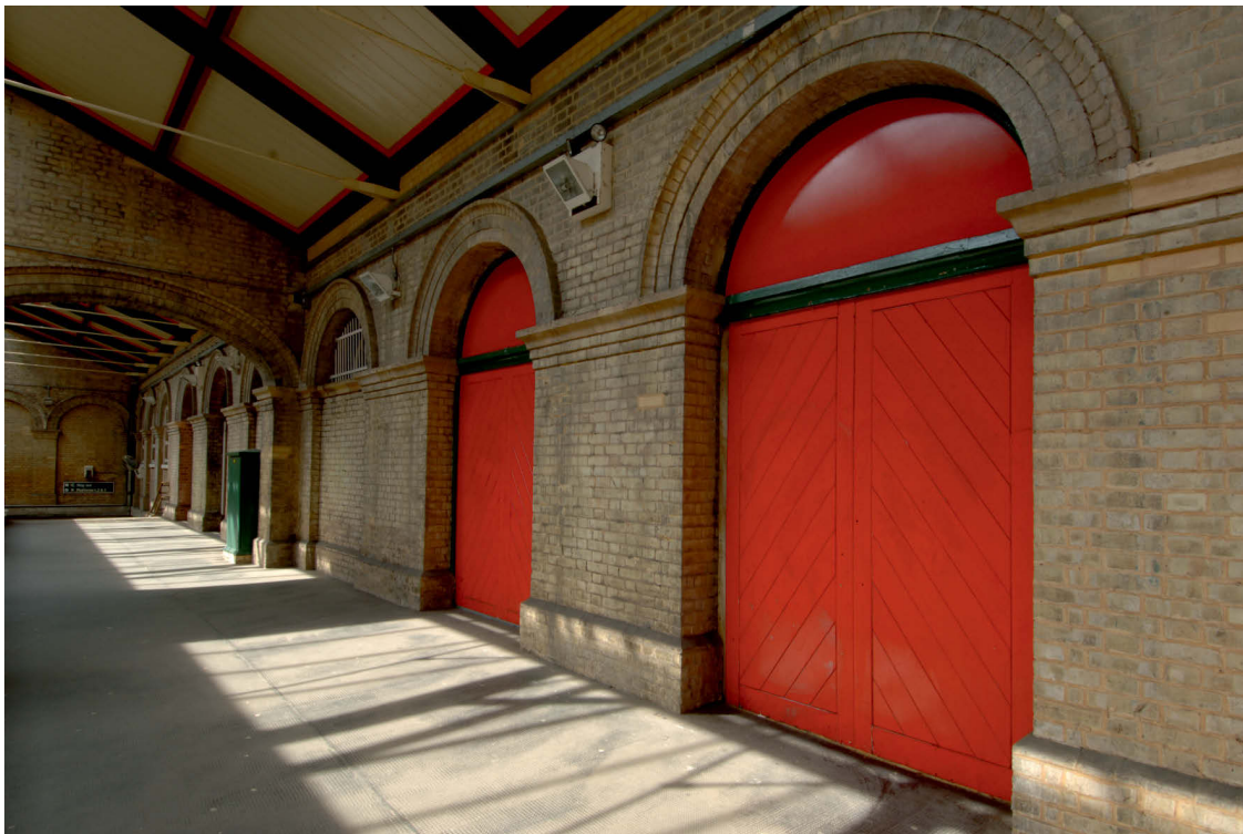
Fig 33 Tasks 16 and 17 with Tasks 14 and 15 in the distance, external view of doorways from ticket hall to platforms, looking south
