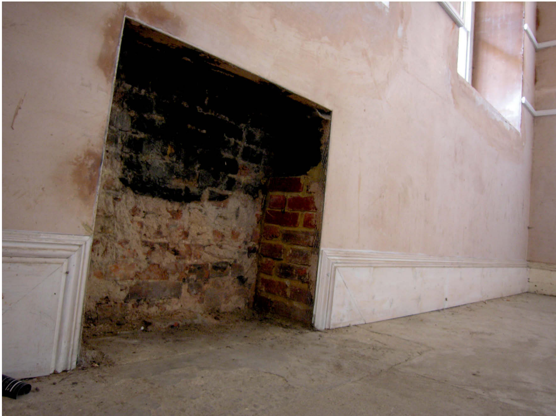
Fig 45 Task 25, detail of the fireplace showing the angled flue, looking south east
