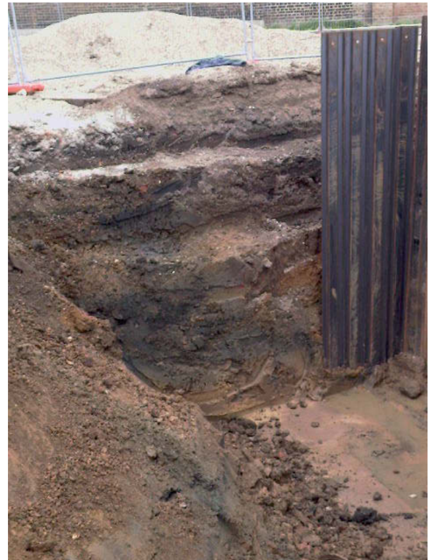
Fig 5 View to southeast in pump room trench, showing grey staining from contamination
