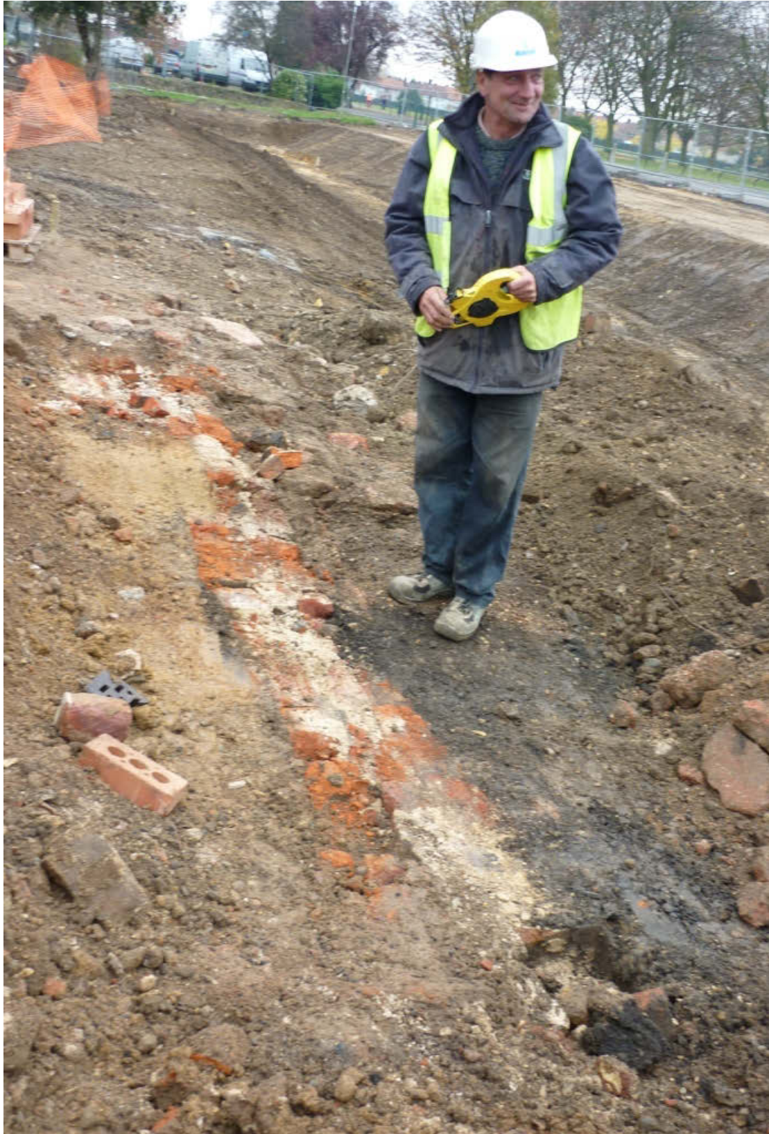
Fig 4 Foundations of old barn exposed in landscaping near to new moat
