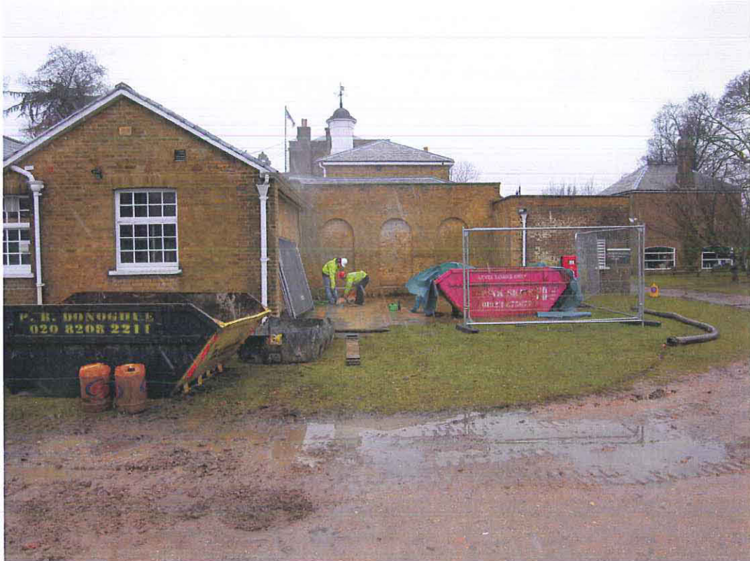
Fig 3 Looking south towards where the extension to the annexe building will be built (ie, the area of foundation trench excavation and borehole drilling)
