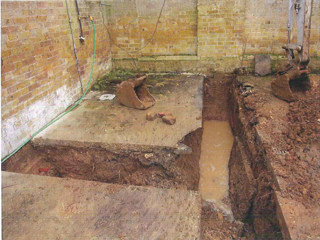
Fig 5 Looking south, showing the foundation trenches excavated to the west of the annexe building (and north of the stables block)
