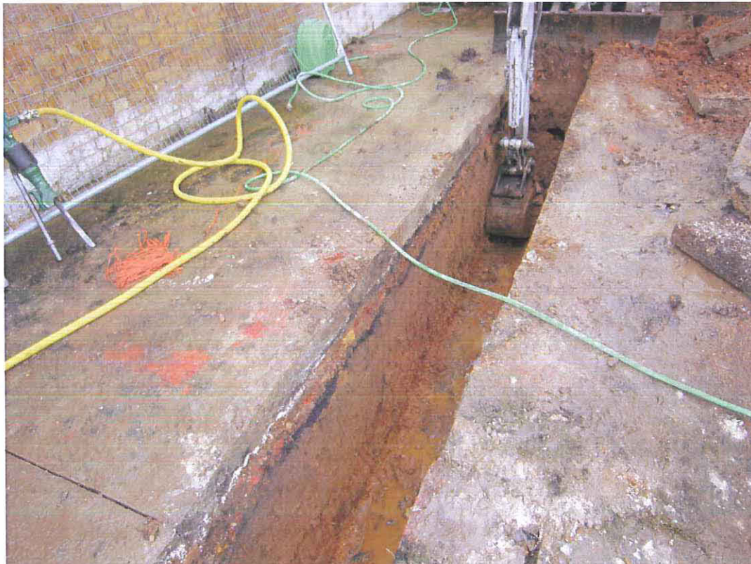
Fig 4 Looking south-east, showing excavation of the north-south foundation trench to west of the annexe building
