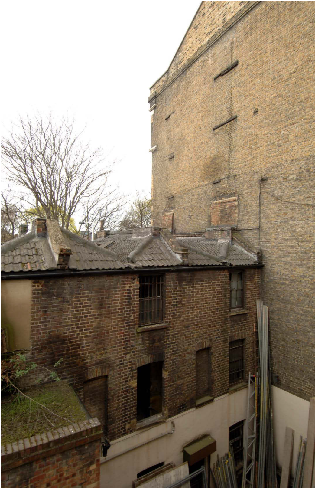
Fig 10 Detail of the metal brackets on the elevation of 239 Long Lane, looking south-west
