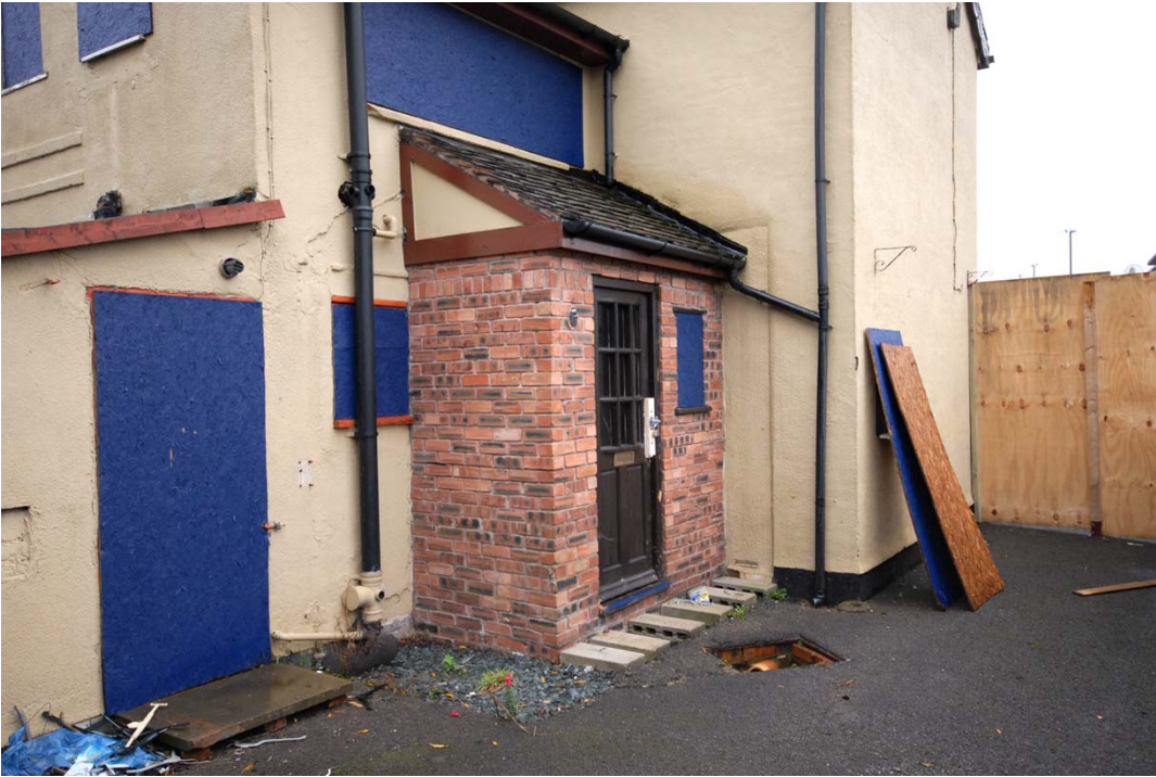
0087 The existing porch and the scars of its larger predecessor Fig 25
