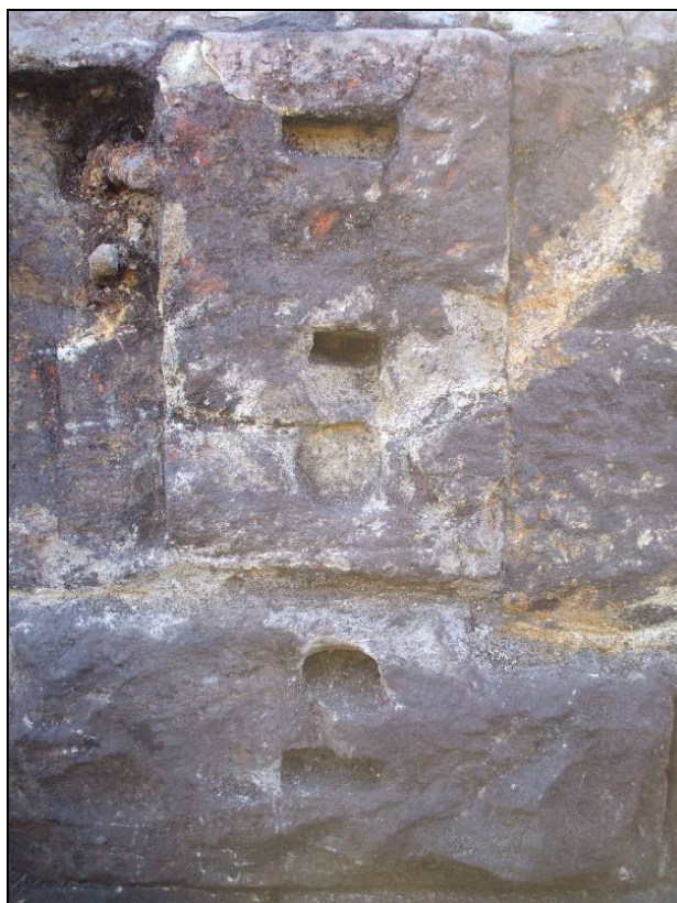
Iron pegs and sockets in west face of culvert/wheel pit wall [1001] Fig 9
