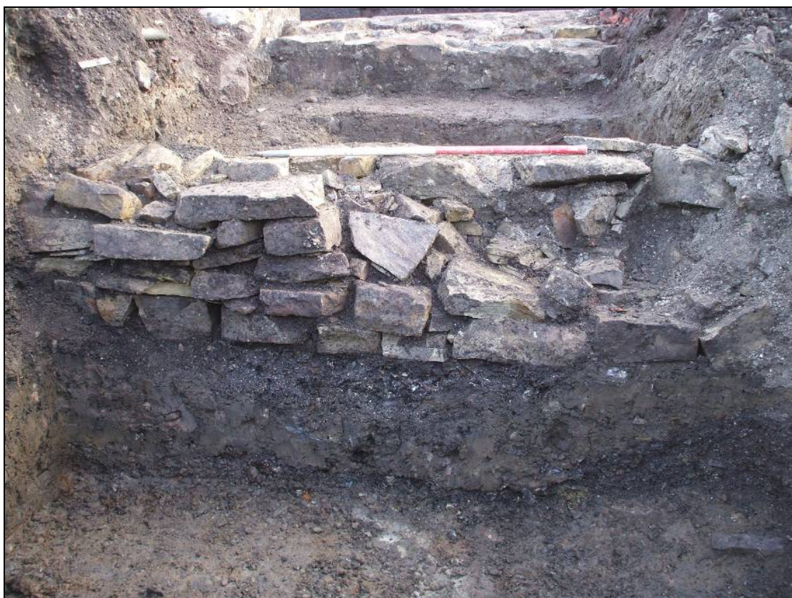
Foundation [2013] for west wall of early 19th-century (?) factory building, looking east Fig 14
