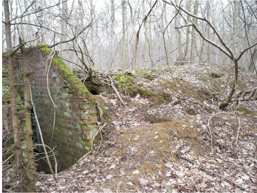
A view of the underground structure located in Area 1, looking north-west Fig 9
