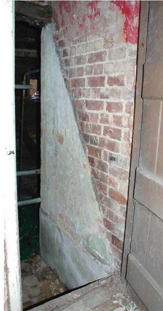
2996 Plaster scar denoting former stair from G15 to F13 ...
