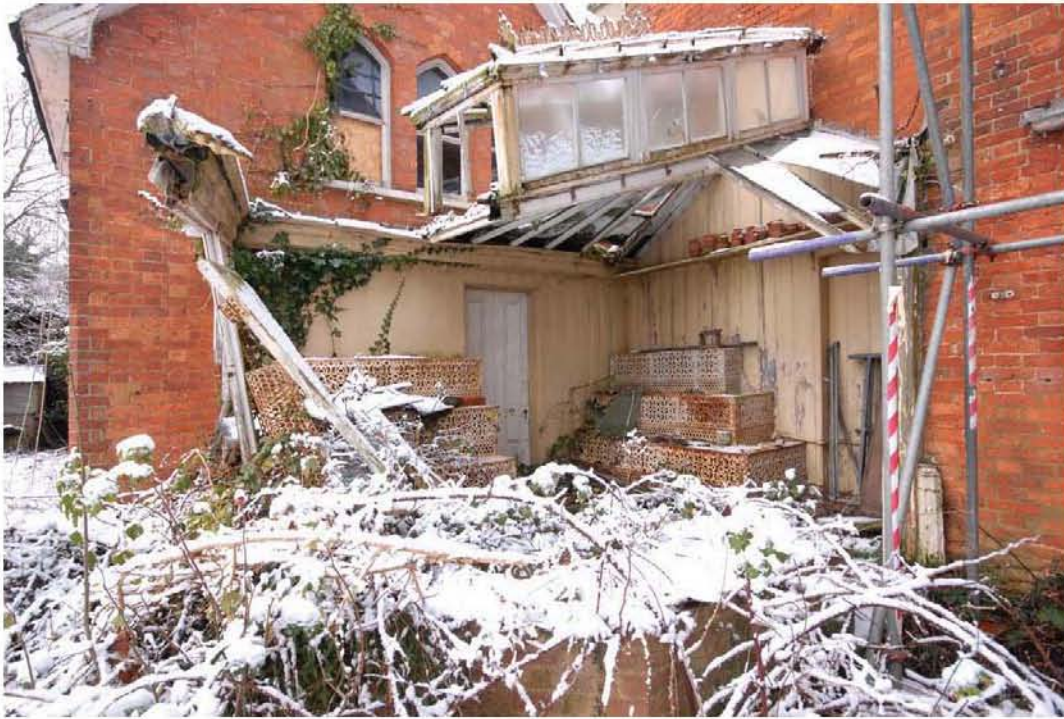
0081 Collapsed conservatory superstructure G18 Fig 61
