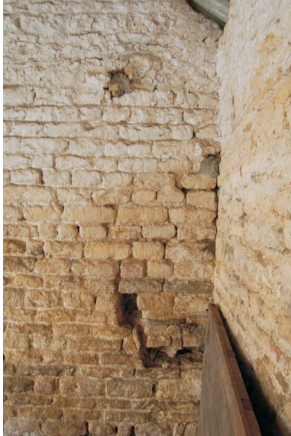
Former location of hayrack and manger in north wall of stock hovel Fig 20
