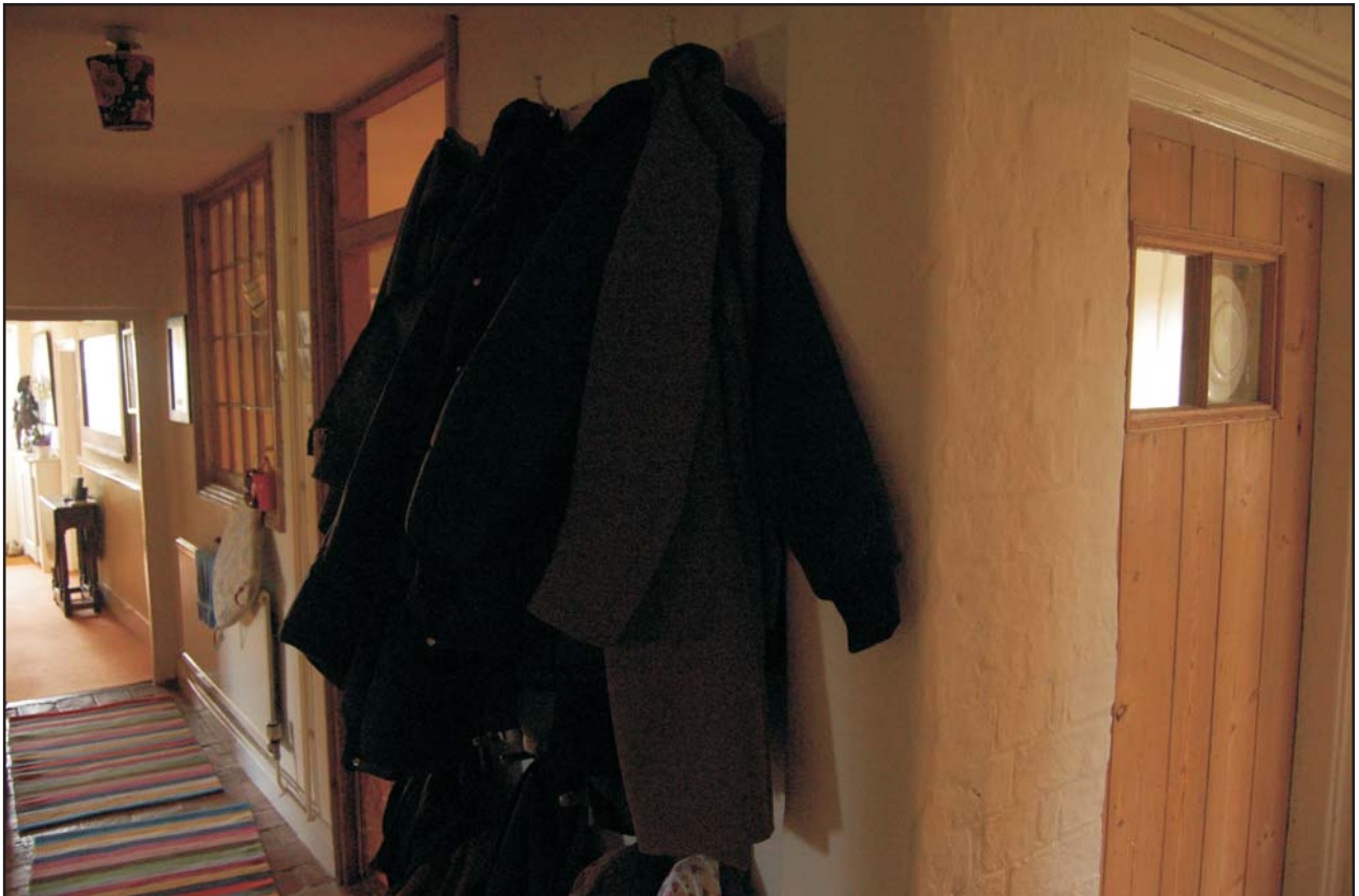
View along corridor G4 at its corner; front of the house to the left Fig 20
