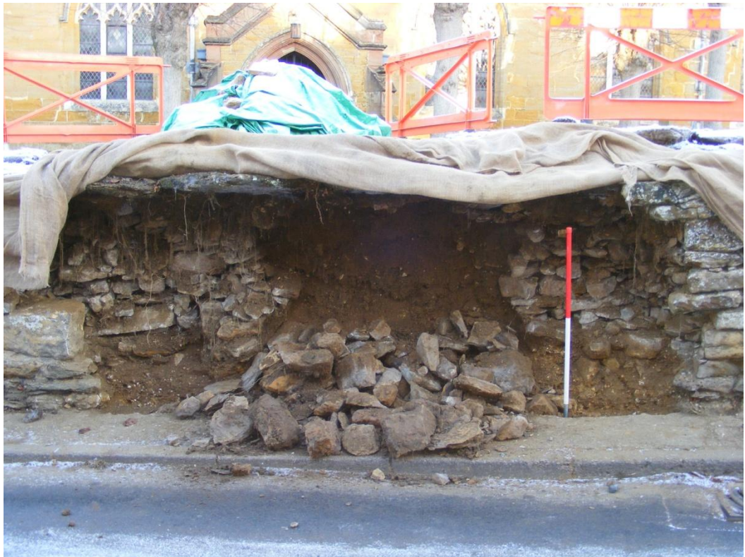
Collapsed retaining wall, looking north Fig 3
