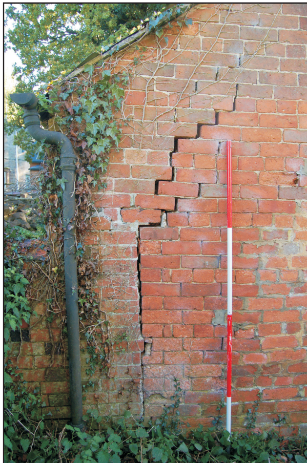
The north wall of the hovel, looking south, showing structural failure Plate 4
