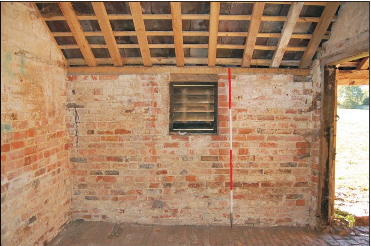
The west internal wall of the southern room with louvred window, looking west Plate 7
