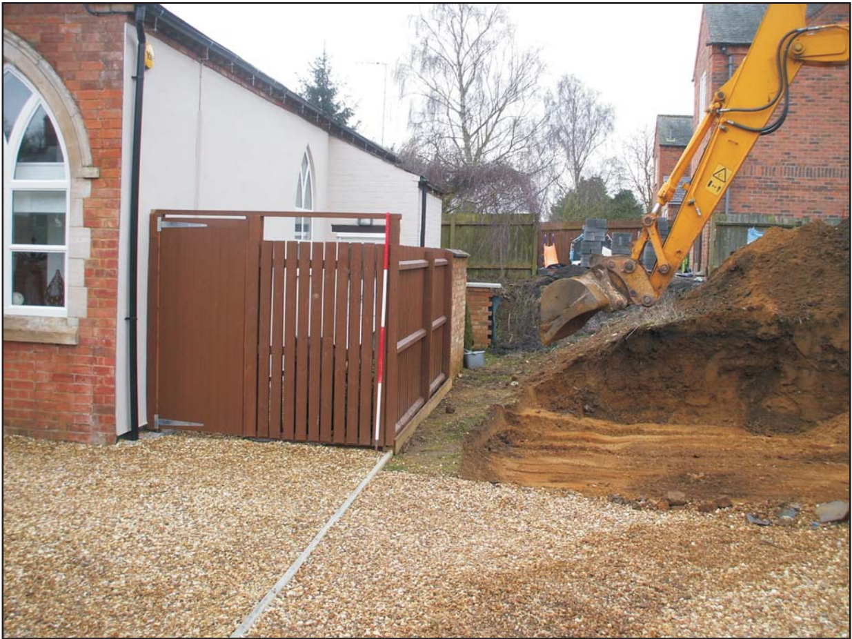
View of the western elevation of the Congregational Church in relation to the development area, looking south-west Fig 8
