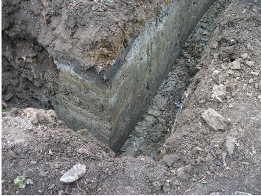
Foundation trench for new house, looking south-east, showing natural clay, right, and backfilled cellar of former cottage, left Fig 4
