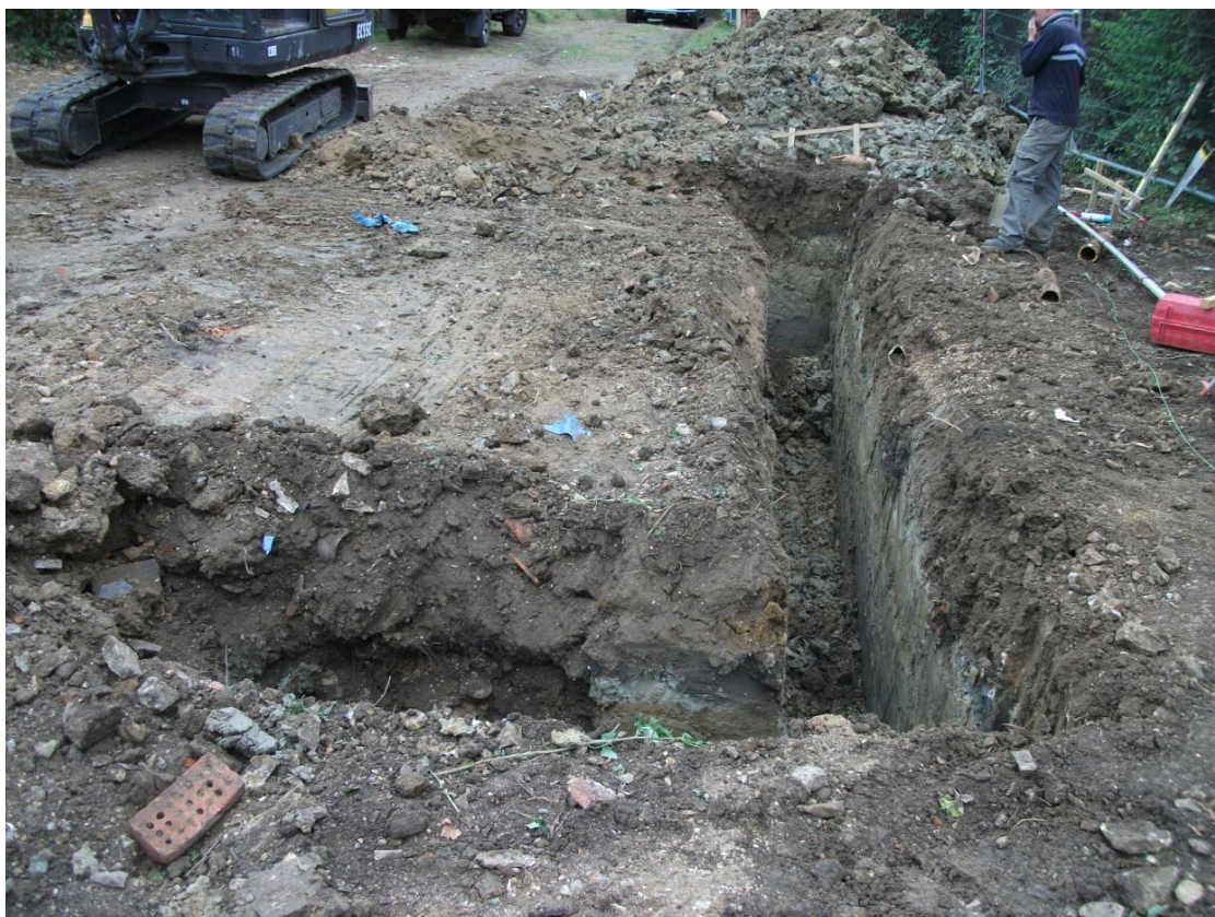
Excavation of the foundation trench for the west wall of the new main house, looking south, showing natural disturbed by drains, right Fig 3
