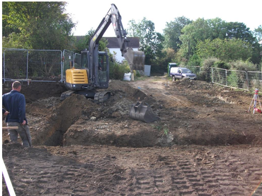
General view of foundation trenches at the northern end of the house extension, looking south Fig 5
