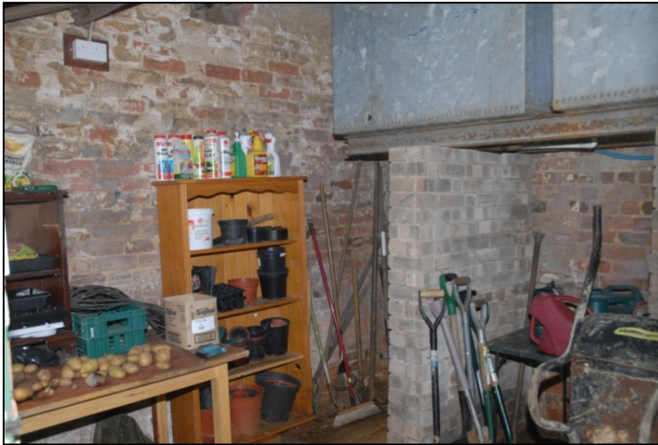
General view of Room 4 showing the water tanks, looking south-west Fig 15
