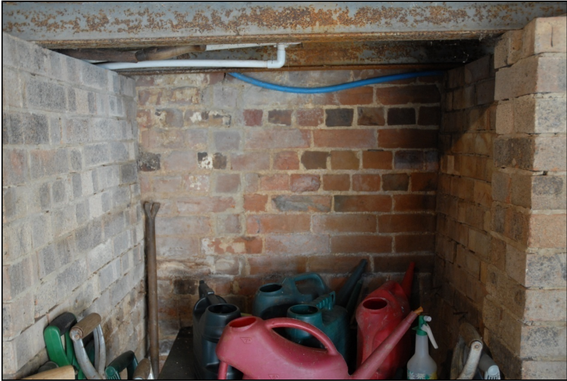
The merging of the older fabric and later rebuild, beneath the water tanks, west wall of Room 1, also showing brick plinths Fig 17
