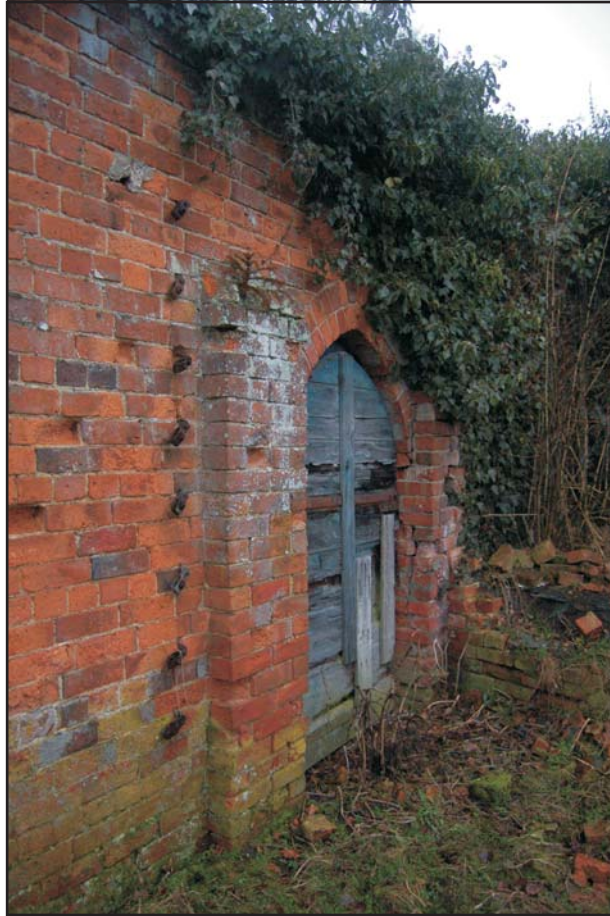
Straining bolts for the cordon wires on the south side of the north wall of the gardens, looking east Plate 13
