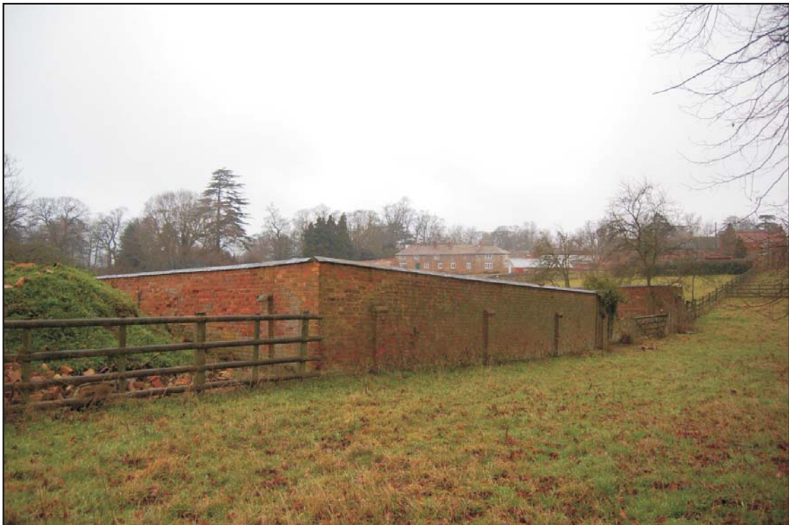
Collapsed section of the south wall (right of photo) from the south-west Plate 8
