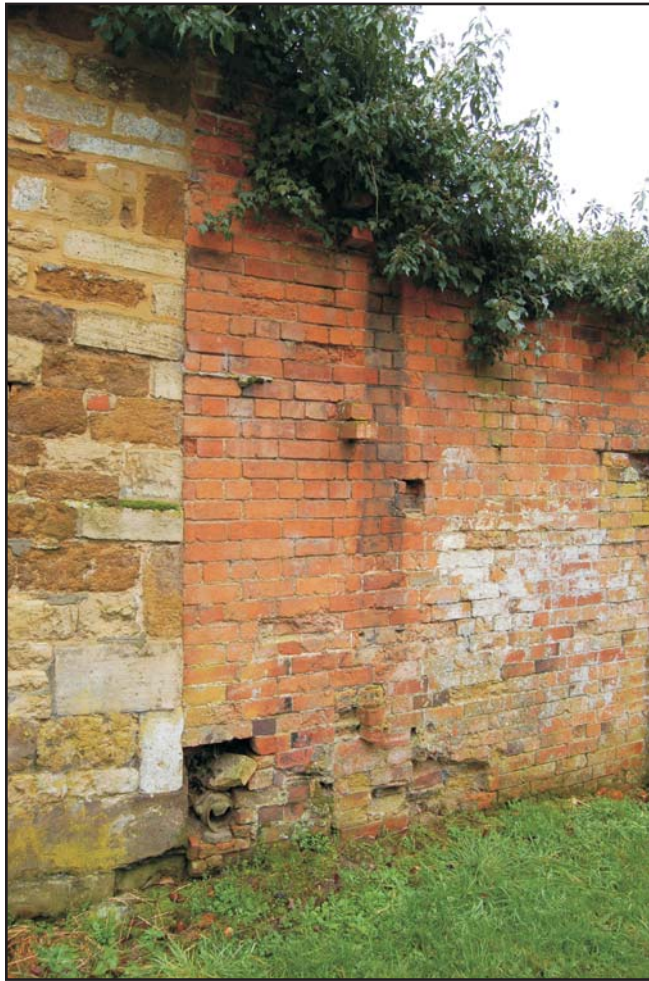
Join of the earlier ironstone faced walled garden, and the later, brick addition, looking south-west Plate 3
