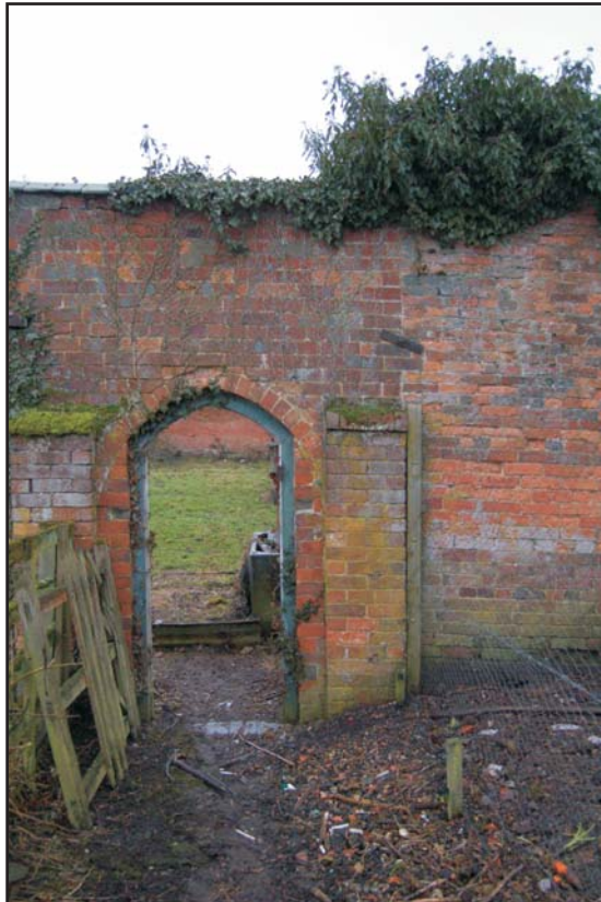
East side of the doorway between the larger and smaller compartments of the walled garden, looking west Plate 12
