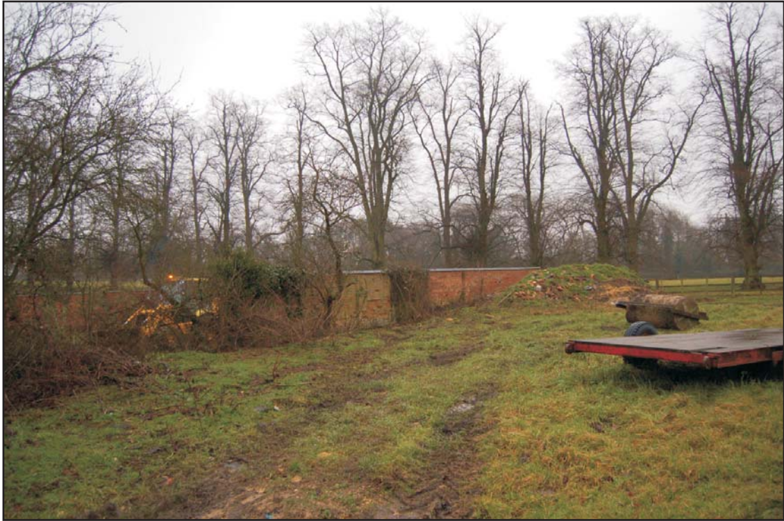
South end of the collapsed west side of the garden, looking south-east Plate 9
