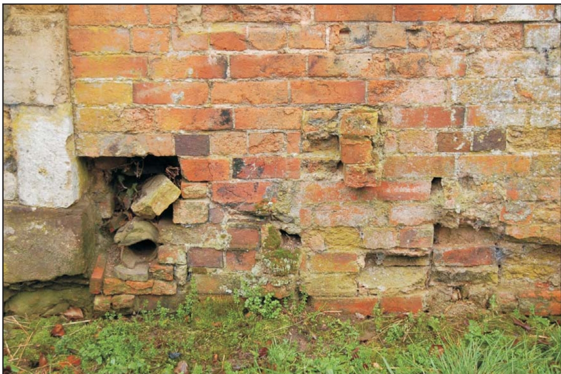
Remnant of cast iron heating pipe within duct from demolished boiler house on north side (foreground) of the garden, looking south Plate 18
