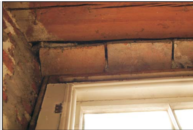
Victorian quarry tiles wedging Library west sash window Fig 5
