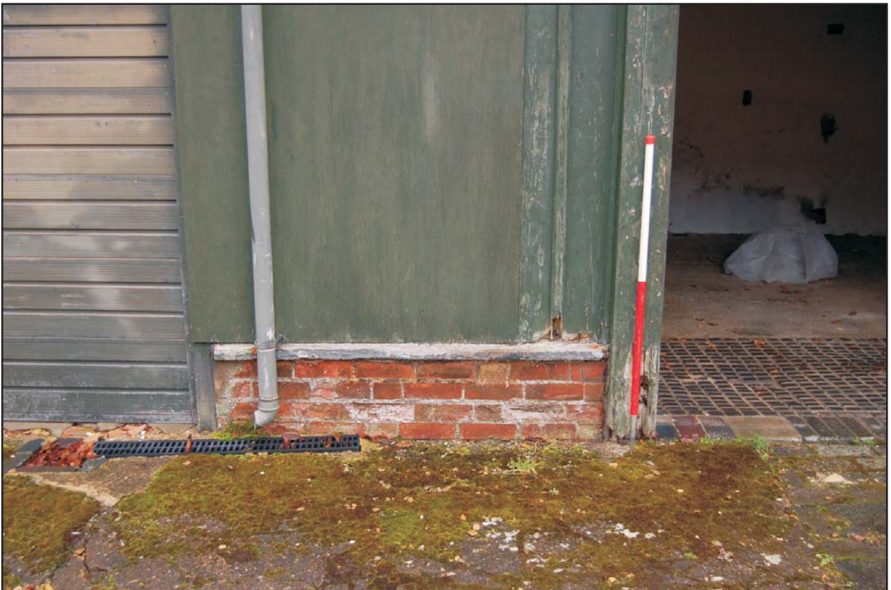
West side showing dwarf Fletton brick wall with timber sole plate Plate 3
