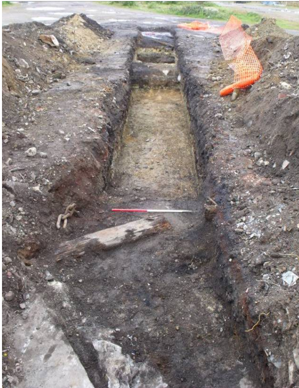
Trench 11 looking north, with the crane base and mooring chain in the foreground (Scale 1m) Fig 30
