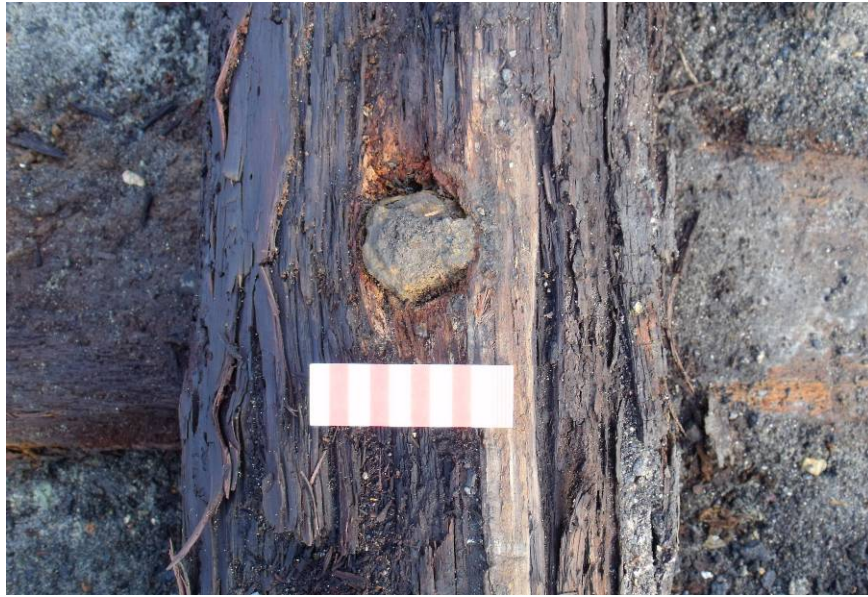
Detail of bolt head joining the timber crane base (Scale 100mm) Fig 23
